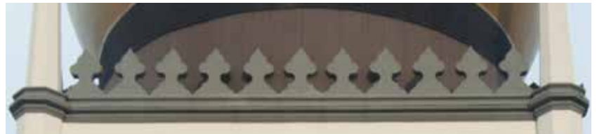
Plaster details cleaned, restored and repainted in new scheme with consideration of maintenance
