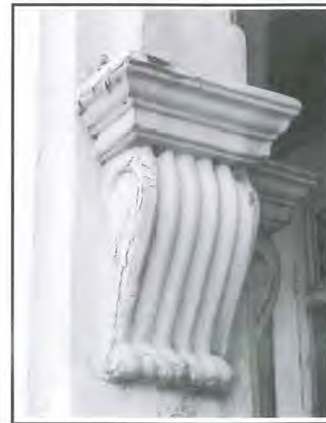
Fig 18: The peeling of paintwork due to excessive layers of paint.
