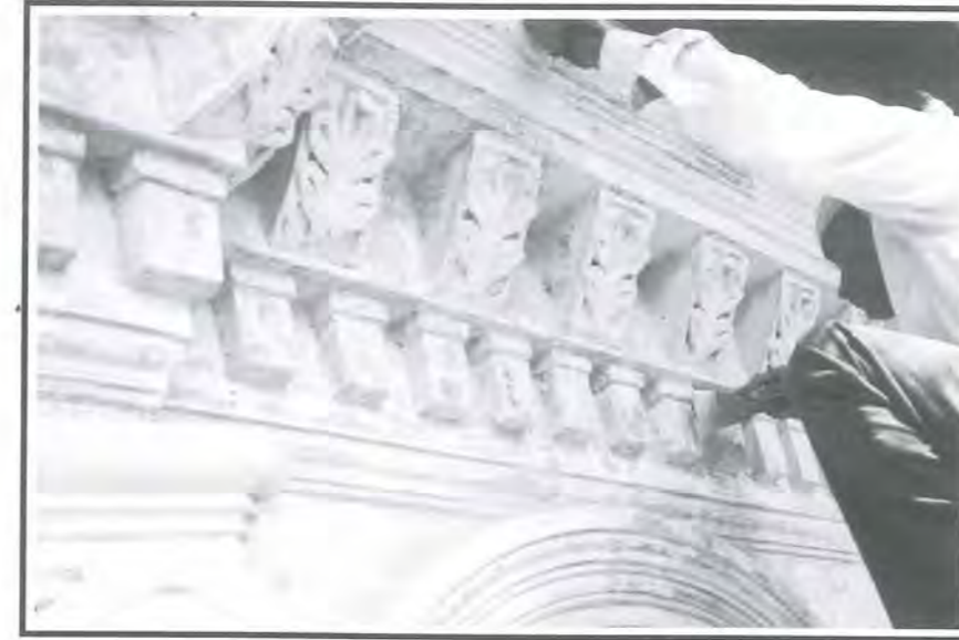
Fig 35: The process of cleaning with light scraping to prepare the surface for repainting.
