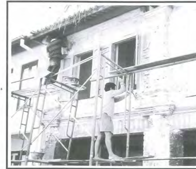
Fig 28: Damaged or decayed plaster in the process of being removed.
