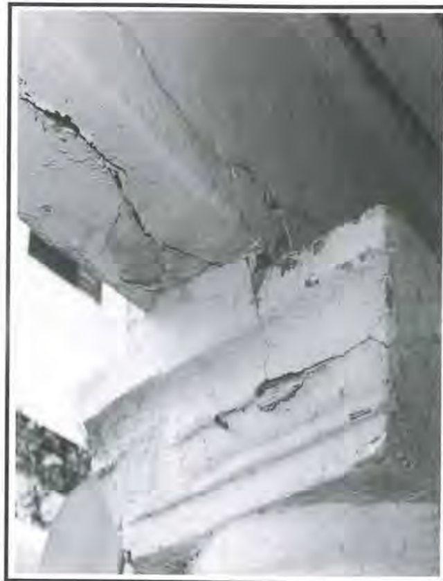
Fig 23: Cracks in the facade beams requiring the need for careful repair before repair of ornamental plasterworks can be carried out.
