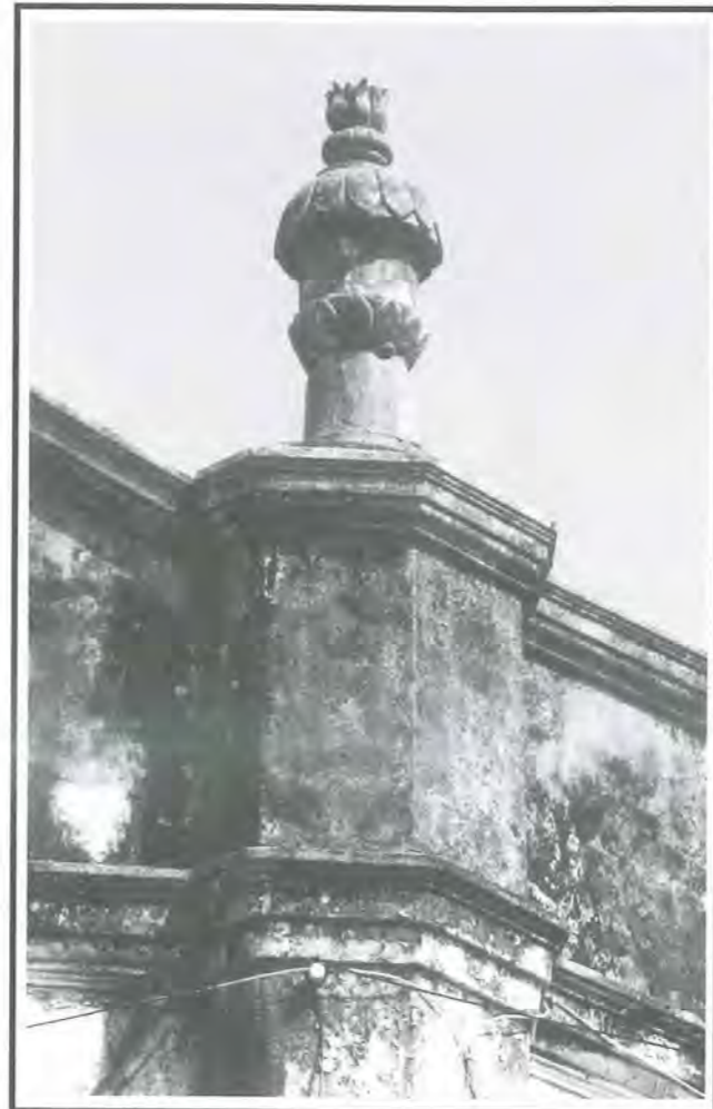
Fig 20: Dampened areas of plasterworks with mosses, lichens and algae growth, requiring the need for biocide treatment.
