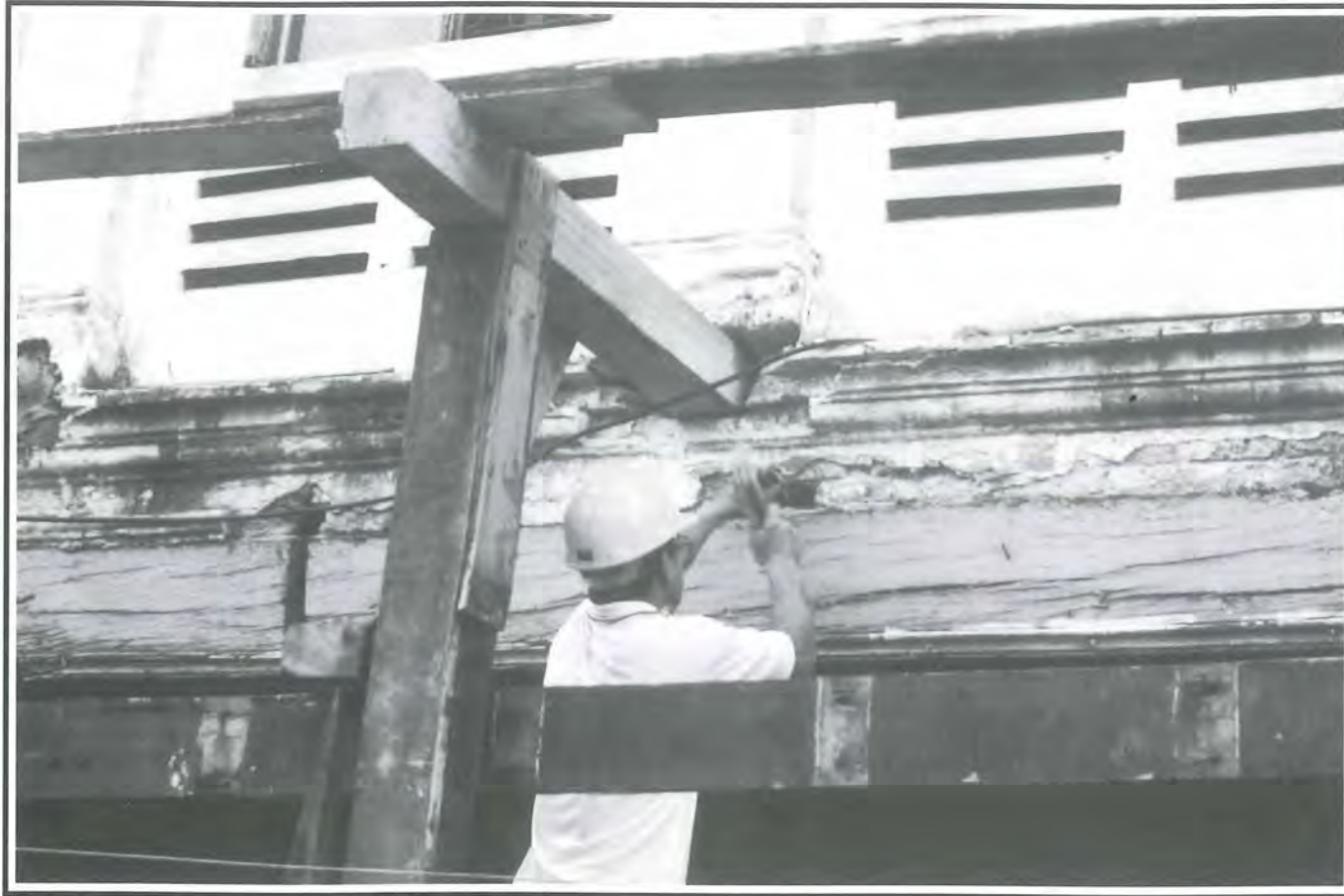
Fig 26: Damaged facade beams in the process of being repaired.
