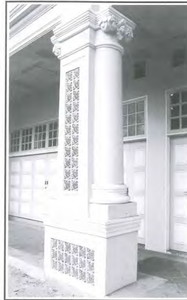
Fig 39: Well-restored column of the Late Shophouse Style. Tile ornamentation and plasterworks reinstated.
