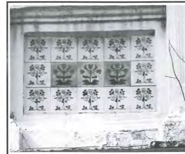
Fig 10: Crumbling of the plasterworks, giving evidence of salt contamination from backing, aggregate or rising damp. This indicates the need for patching repair.
