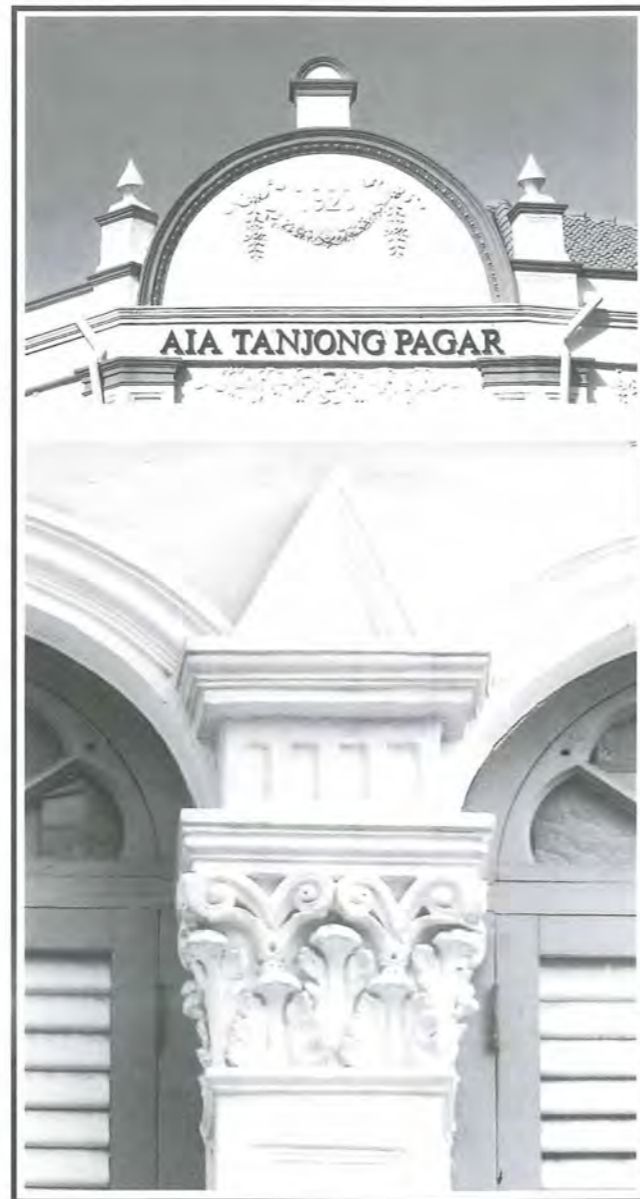
Fig 41: Restoration of the elaborate ornamentation on pediments, arches and columns, bring back to life the craftsmanship of the past.
