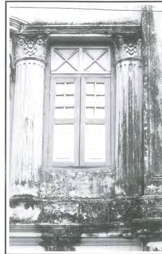
Fig 21: The stained plasterworks due to environmental grime, requiring the need for cleaning with mild abrasive systems like hand brushing and the use of detergents coupled with hot water.
