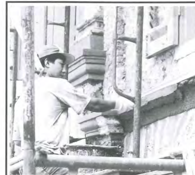
Fig 29: Reconstruction and patching-up of damaged plasterworks on site in the process of restoration.
