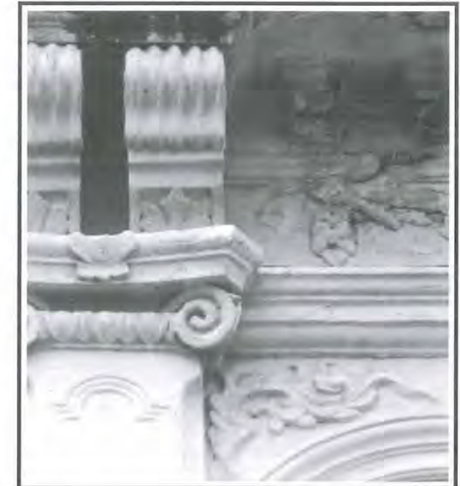
Fig 22: Weathered plasterworks in need of cleaning and repair.
