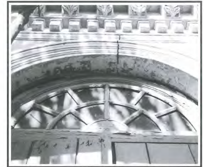
Fig 11: Cracked architrave, indicating the need for in-situ repair works.
