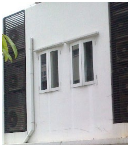
A/C ledges: Louvers with insufficient depth
