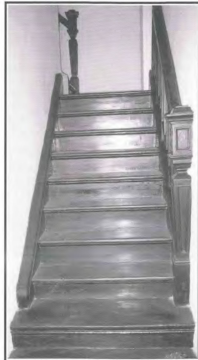
Fig 29: Restored timber staircase to be properly maintained to prevent deterioration due to water accumulation and termite infestation.
