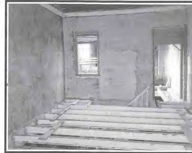
Fig 2: Location of existing staircase is tied in with the existing timber floor structure.
