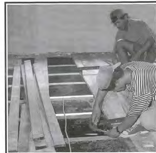
Fig 21: The use of tongue and groove joinery during restoration as a fire-safety measure.
