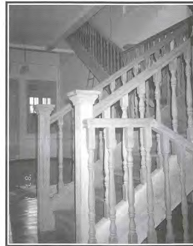
Fig 19: Reconstruction and reconfiguration due to changes in the internal layout of the shophouse.
