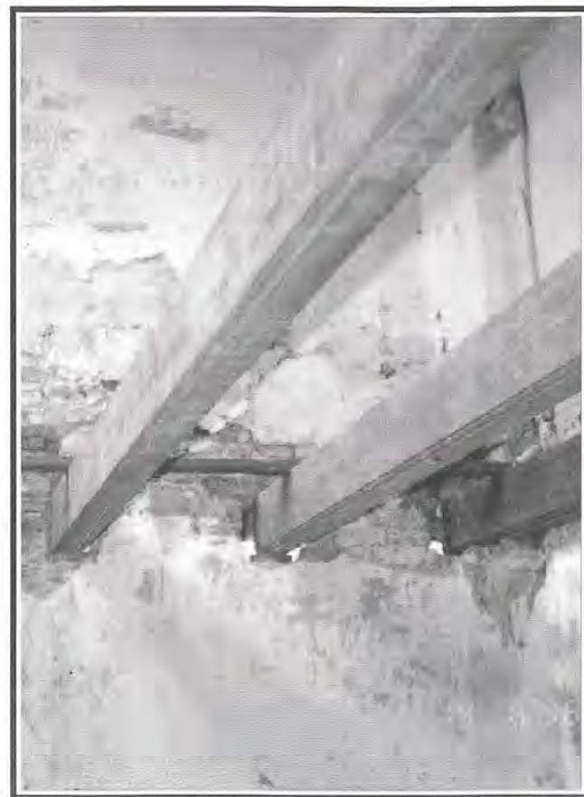
Fig 11: Insertion of additional timber floor joists between the existing joists to reduce the loading on the original members.
