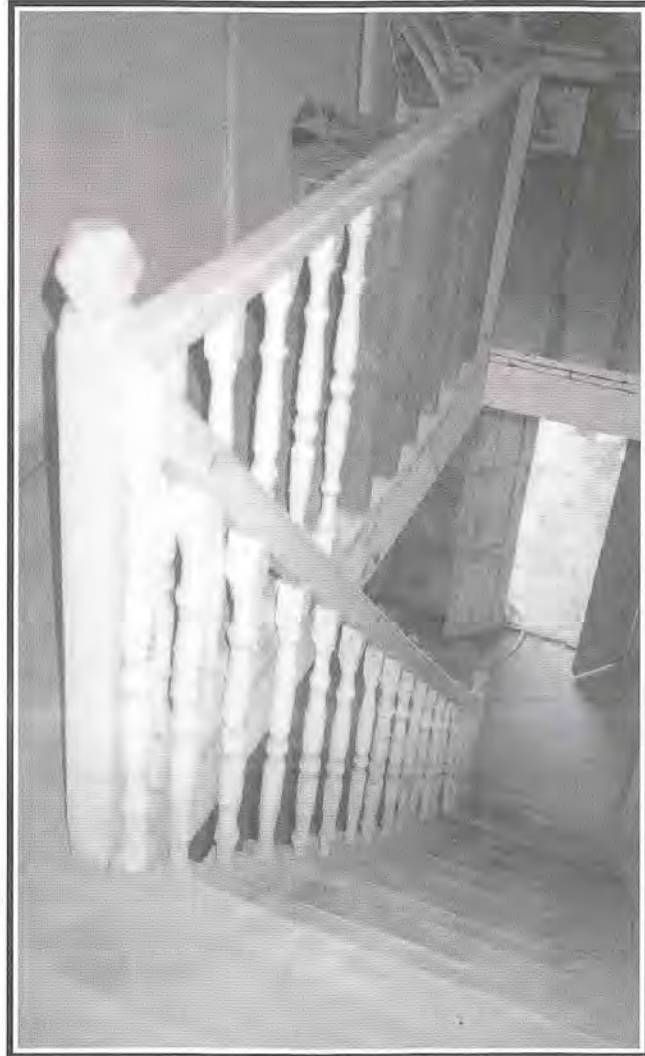
Fig 16: Mismatched balustrades before restoration.
