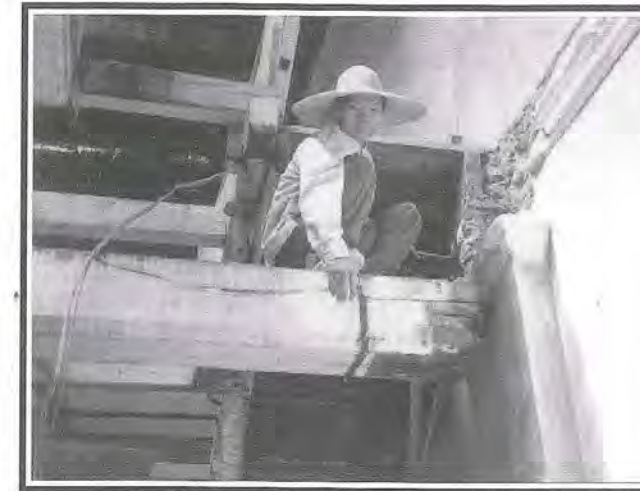
Fig 7: Areas of rot usually occur at the ends of the timber floor structural members.
