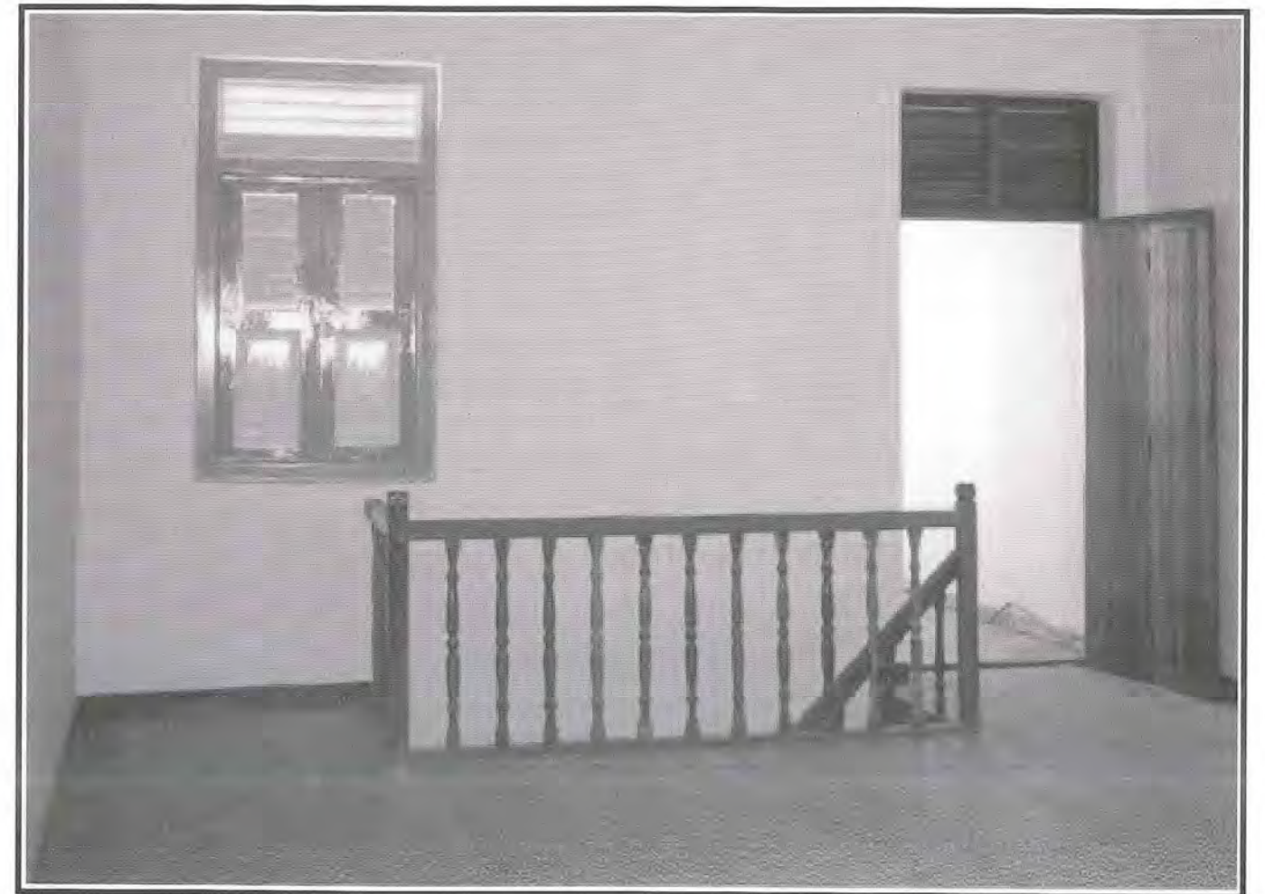
Fig 4: Existing location of staircase retained after restoration. Original spatial quality of shophouse is retained.
