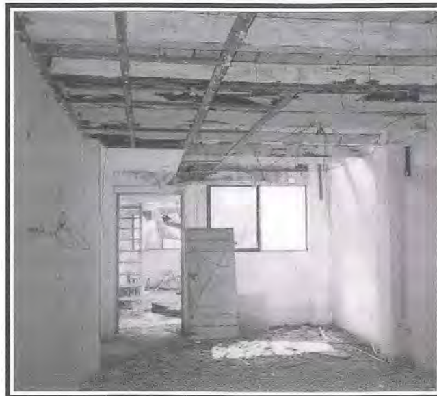
Fig 5: Visual inspection of the timber floor joists and boards should be carried out to determine the extent of decay and structural damage.
