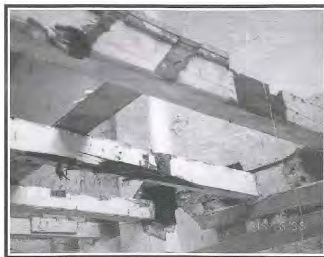
Fig 6: Badly deteriorated timber floor joists due to termite infestation, water penetration and fungal attack.
