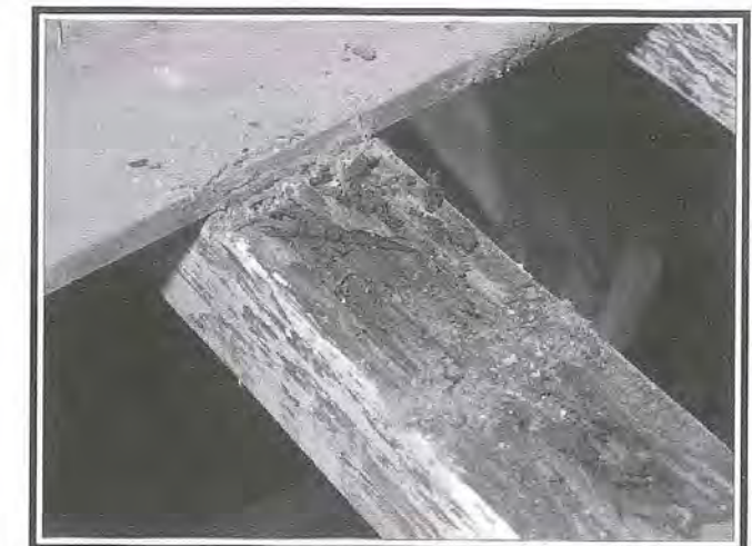
Fig 8: Timber splinters lifted up in short irregular pieces as a result of breakdown of the fibre strength due to timber decay.
