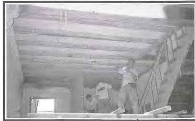
Fig 24: Use of non-combustible boards between timber floor joists to achieve the required fire-rating.
