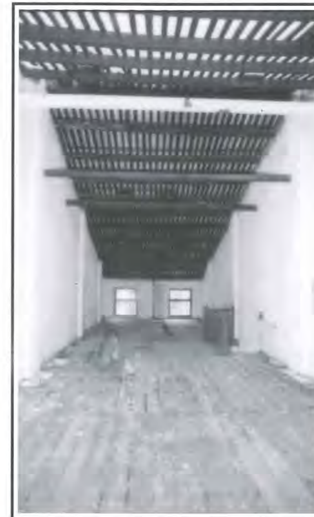
Fig 7: Lateral bracing of the structure, retention of the timber floor boards and joists, and replacement of timber roof purlins on a elemental basis will help to maintain the lateral stability of the partywalls during restoration.
