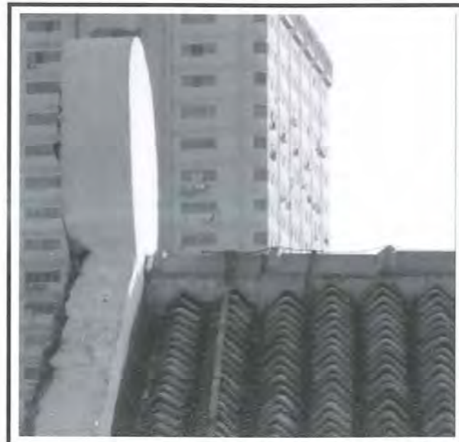
Fig 23: The laying of the lightning conductor along the partywalls and on the ridge of the main roof.
