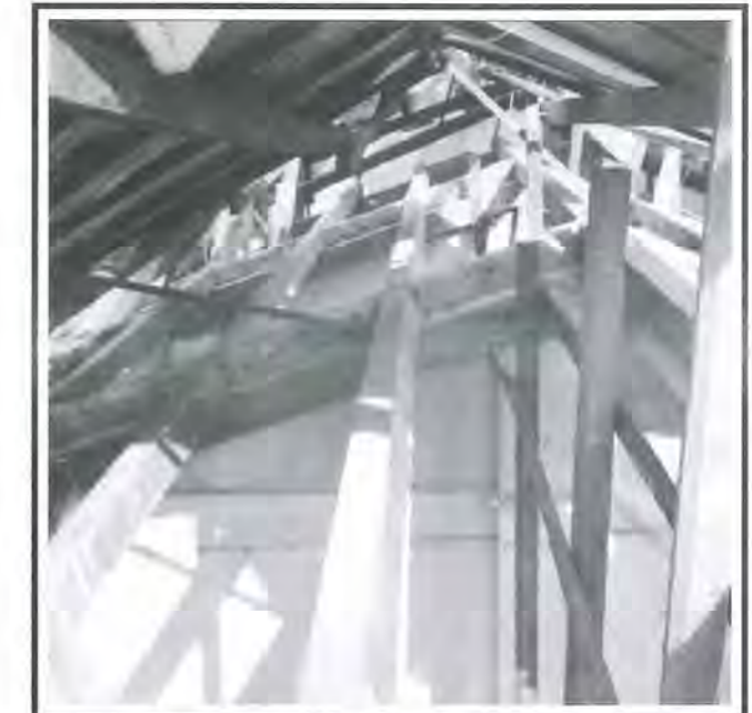
Fig 11: The replacement of the roof timber structure carried out under the temporary protective cover.
