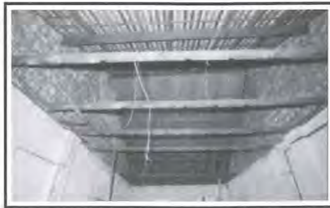
Fig 8: Visual inspection of existing roof support structure should be carried out to determine the extent of decay and structural damage.
