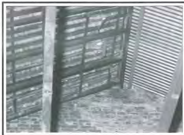
Fig 9: Decayed roof timber members, some of which require replacement while others require strengthening.
