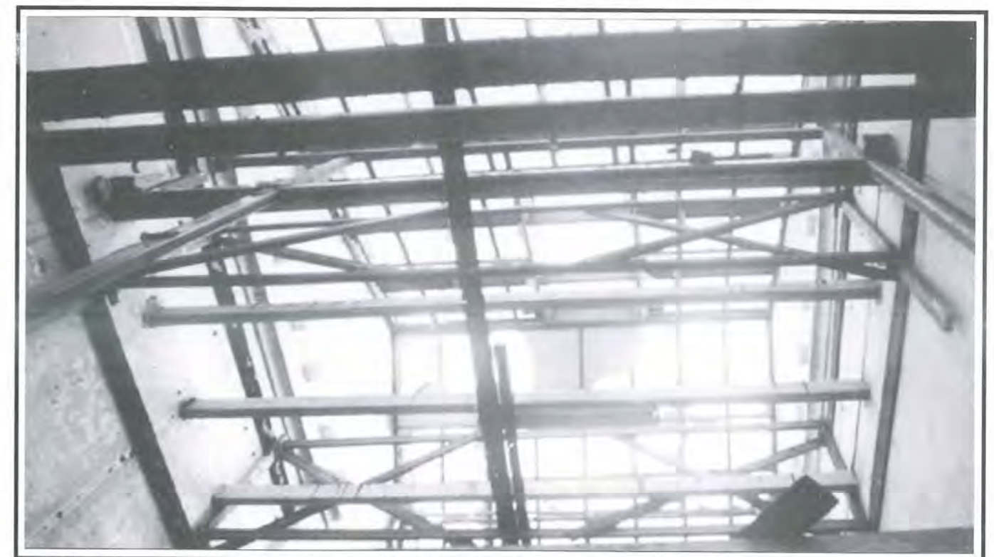
Fig 7: Adequate protection and lateral stabilisation during restoration works would prevent the collapse of the partywalls.
