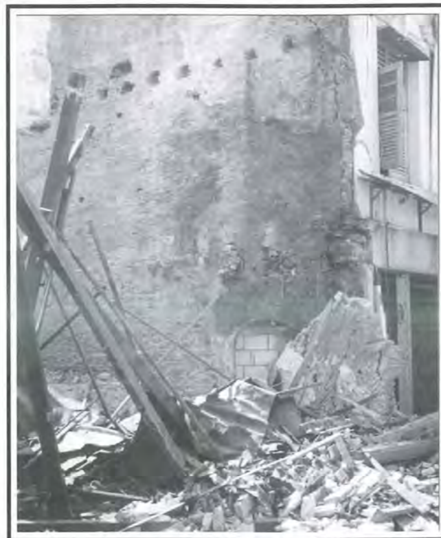
Fig 4: Collapse of partywalls during restoration works is often due to the removal of lateral restraint to walls, lack of provision of temporary support or shoring, improper structural intervention, undermining of existing foundation or structural overloading.
