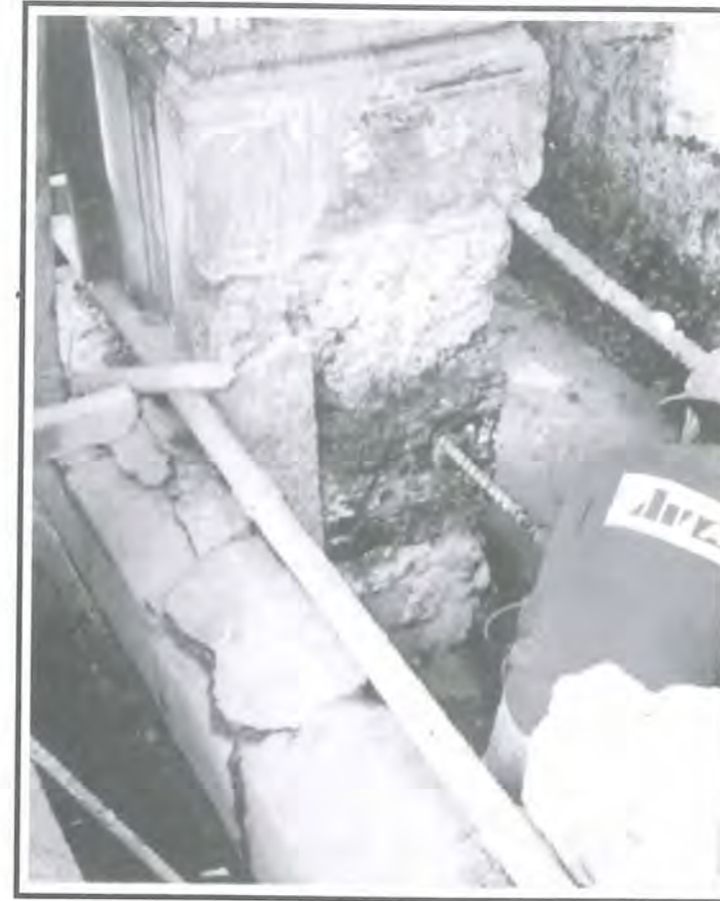
Fig 20: The strengthening of the existing foundation with reinforcement to prevent the collapse of the partywalls.
