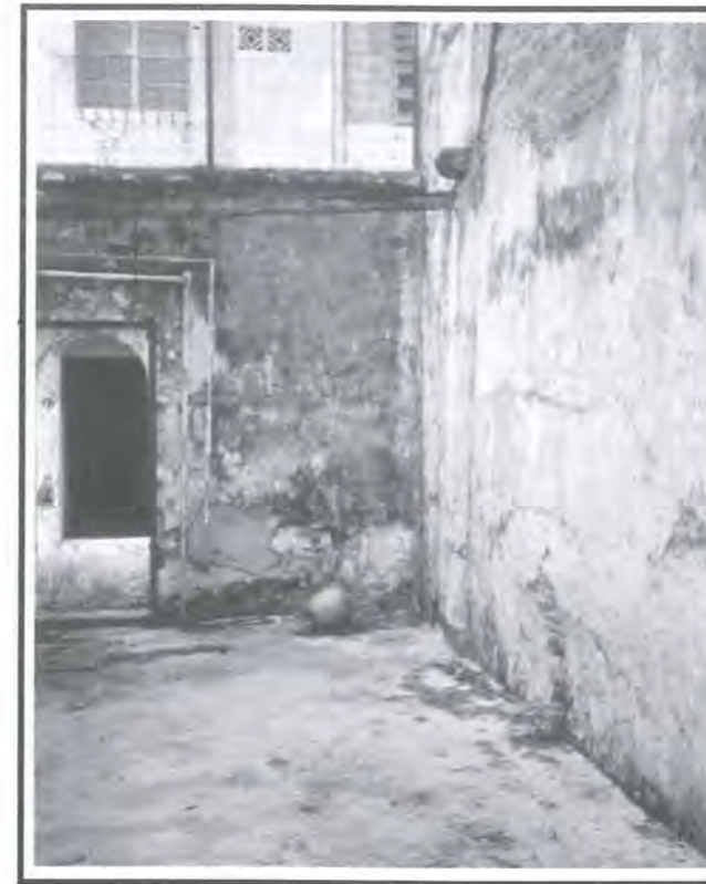
Fig 1: Cracks on the walls, due to weathering or structural settlement, require proper treatment and repair.
