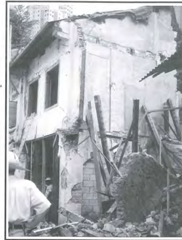
Fig 5: Partywall collapses could also be due to the structural instability of the existing partywalls which could be detected through comprehensive assessment of the existing structure.
