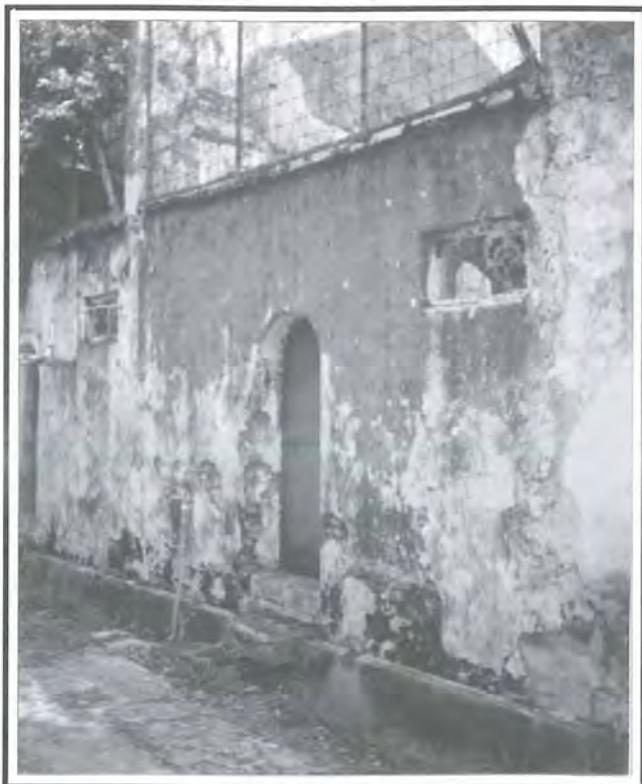
Fig 14: Damage to the plaster rendering arising from the loss of adhesion due to water penetration or crumbling, and powdering on the surface as a result of salt contamination from backing, aggregate or rising damp.
