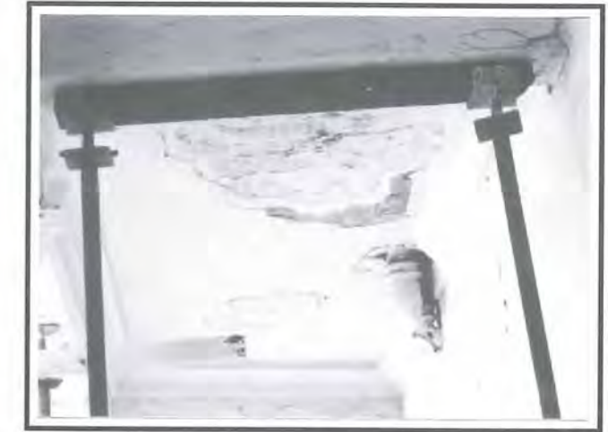
Fig 6: Propping up of the decayed timber beams during restoration is a means of providing structural stability.
