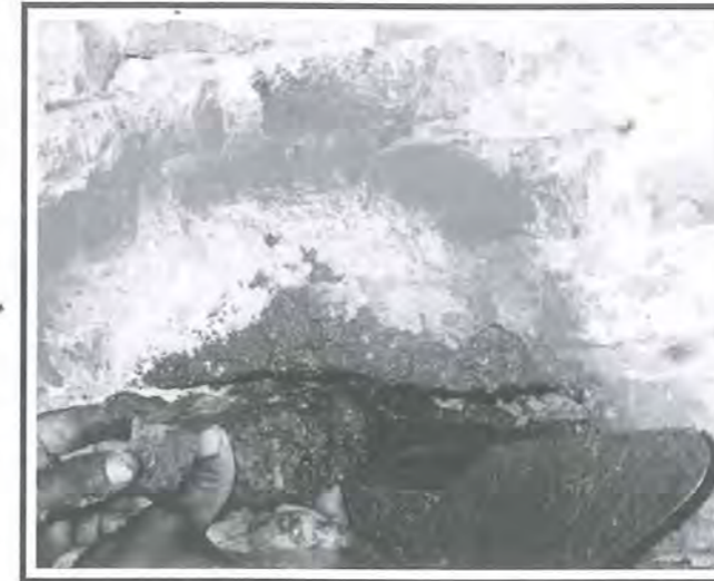
Fig 9: The process of stitching of new bricks and mortar jointing as a means of localised repair to the old brickwall.
