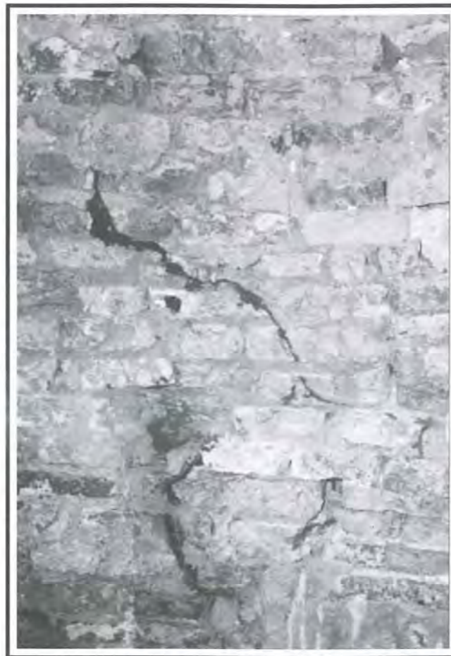
Fig 8: Cracks in existing brickwall indicate damage to the old bricks, thereby requiring areas of localised repair.
