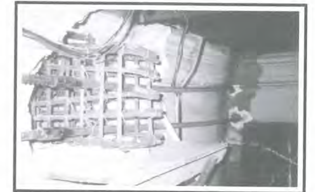
Fig 22: The addition of new reinforced concrete beam in an existing partywall as a means of structural intervention.
