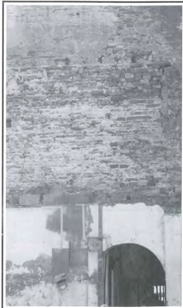
Fig 15: Parts of the brickwall, upon removal of the existing plaster rendering, require localised repair.
