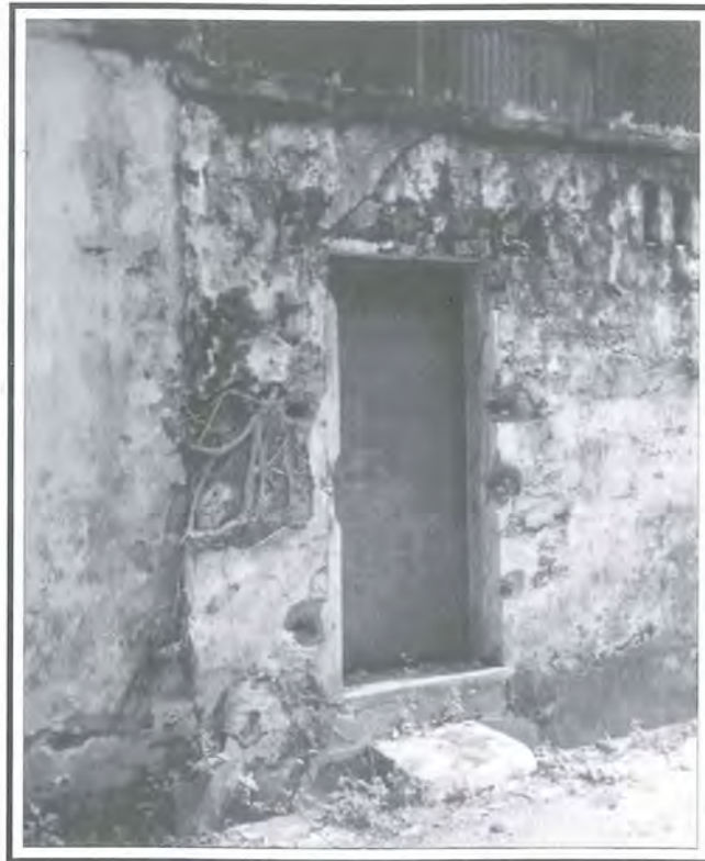
Fig 13: Damage to the plaster rendering due to vegetation growth and water penetration.
