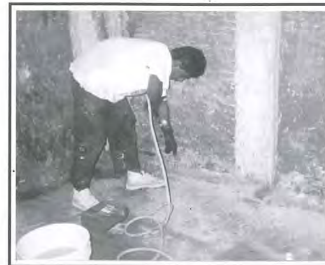
Fig 10: The process of injection of silicon into the brickwall to prevent water penetration through capillary action from the ground.
