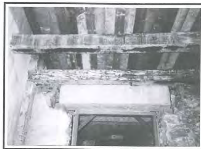
Fig 19: The use of concrete lintels for the creation of openings in the partywalls for amalgamated units.
