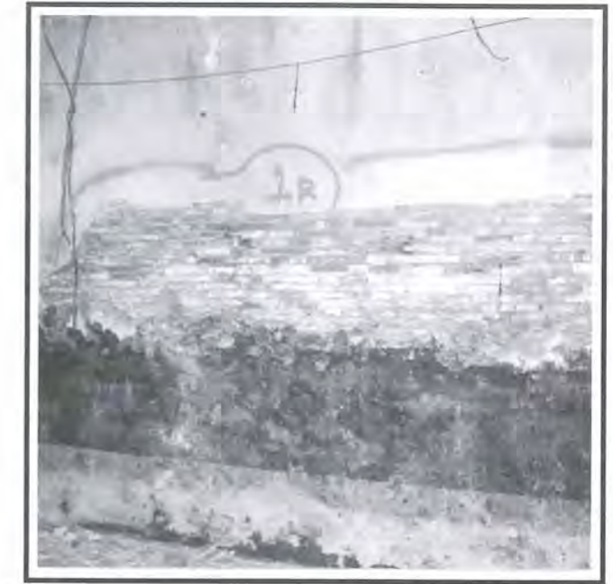
Fig 2: Organic growth on the partywall, caused by water penetration and the humid environment, requires proper treatment and cleaning.
