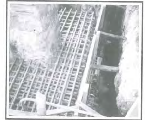
Fig 21: The addition of reinforcement to the existing reinforced concrete columns and ground structure to increase the loading capacity of the structure.
