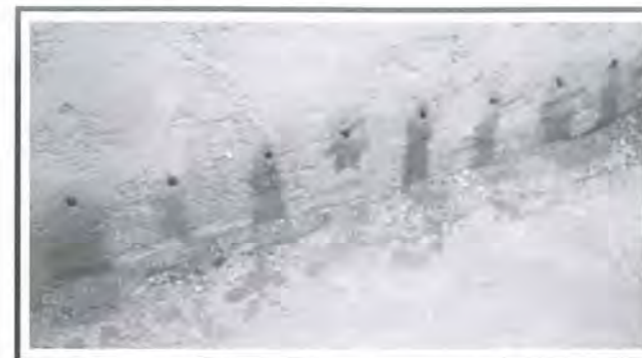
Fig 11: The holes made at about 500mm above the ground for the injection process.
