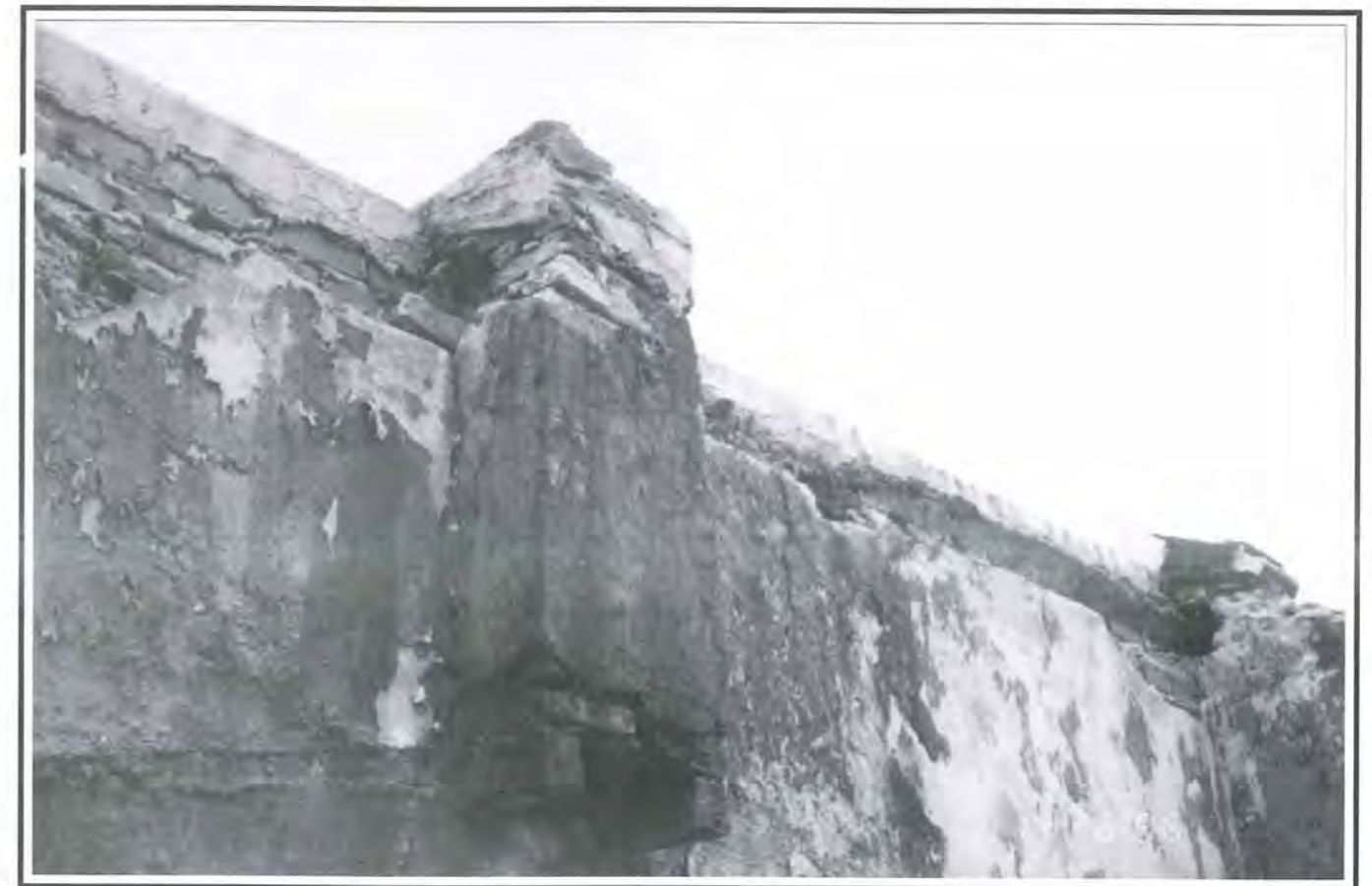
Fig 3: Deteriorated partywall, due to algae, moss and lichen growths, requires proper treatment and repair.
