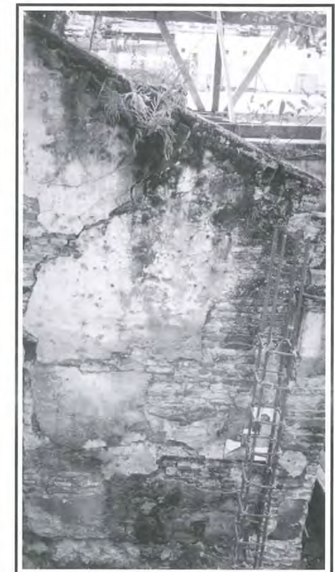
Fig 12: Cracks and areas of localised damage of the existing plaster, require proper cleaning, repair and treatment.
