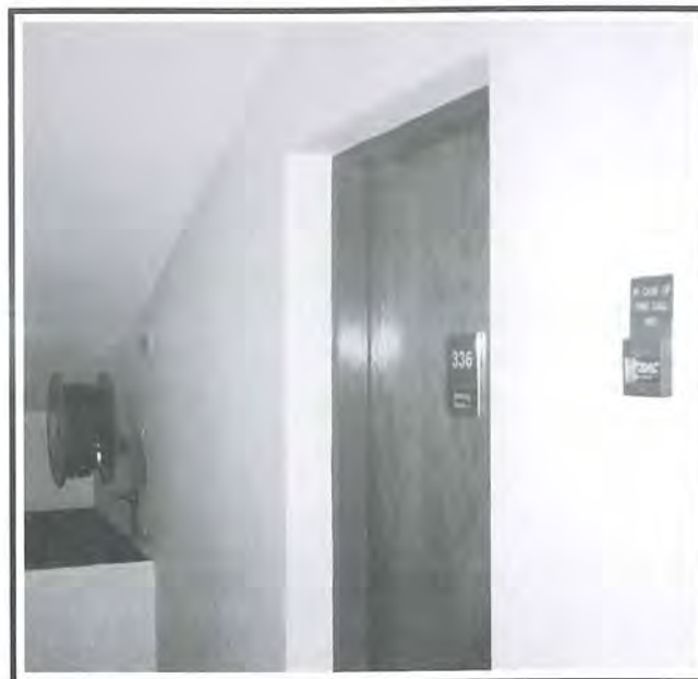
Fig 17: A hosereel is necessary for a compartmented attic floor.
