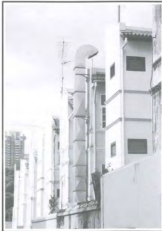
Fig 12: Unsightly exposed flue which mars the rear elevation of the conservation building.
