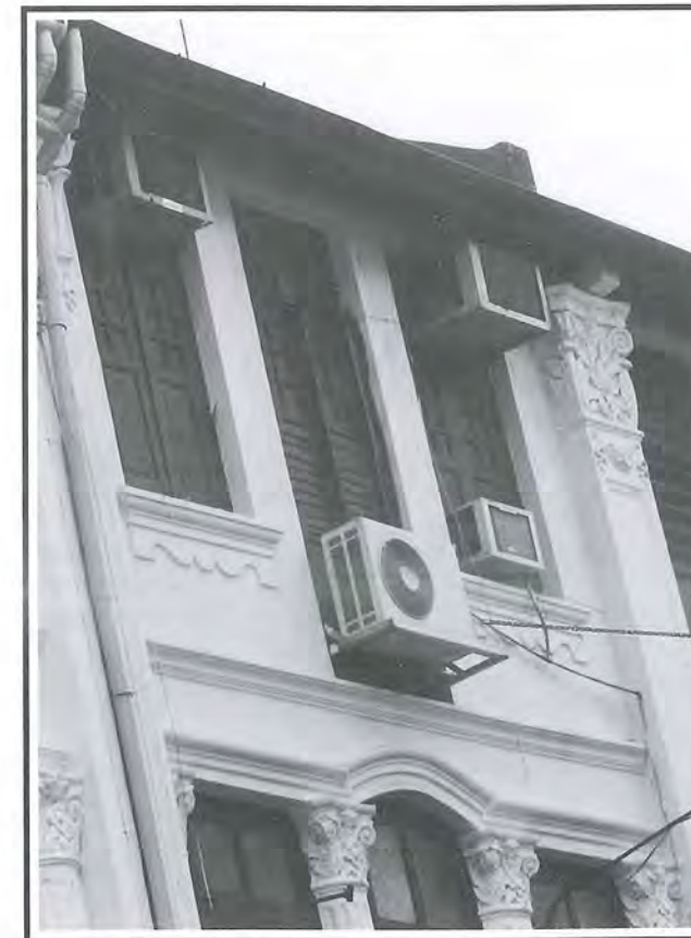
Fig 8: Window air-condensing units should not be used as they mar the facade of the conservation building.
