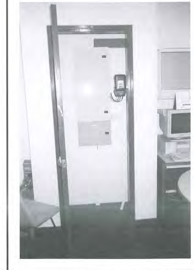
Fig 2: Electrical meter and telecom distribution board positioned within a niche in the wall and well concealed by a timber louvred door.
