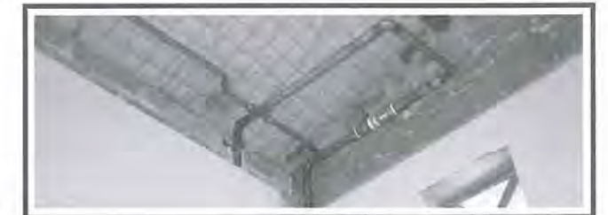
Fig 3: Pipes installed above the false ceiling.
