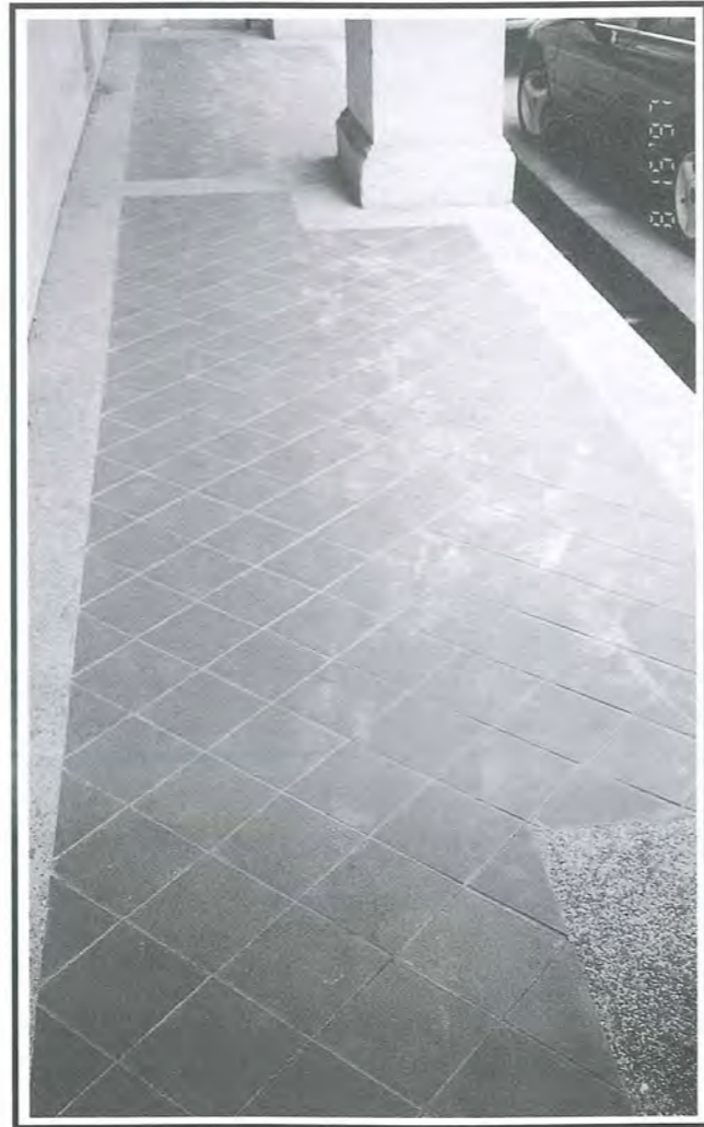
Fig 9: The use of terracotta tiles with granite edging is also commonly found.
