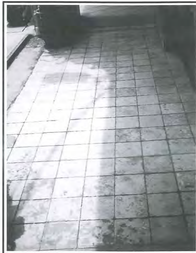
Fig 25: Minor repair works and cleaning are required for this cement floor finish.
