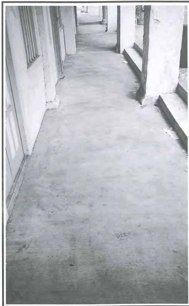
Fig 7: The use of plain cement screed along the five-footway are typical of the earlier shophouse styles.
