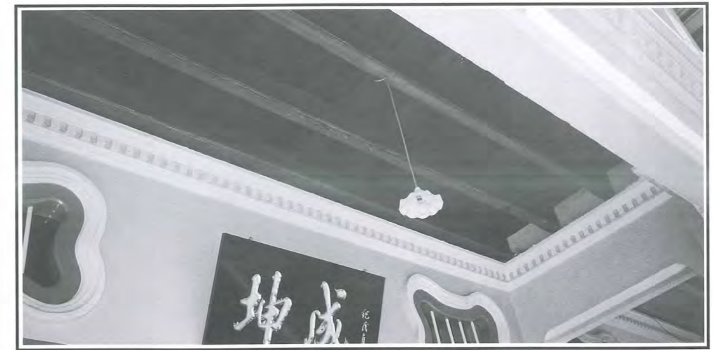
Fig 11: Exposed underside of the upper floor timber joists and floor boards enhanced by elaborate cornices.
