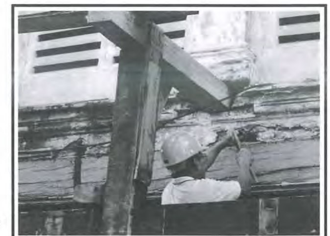
Fig 30: A deteriorated front facade timber beam in the process of being strengthened.
