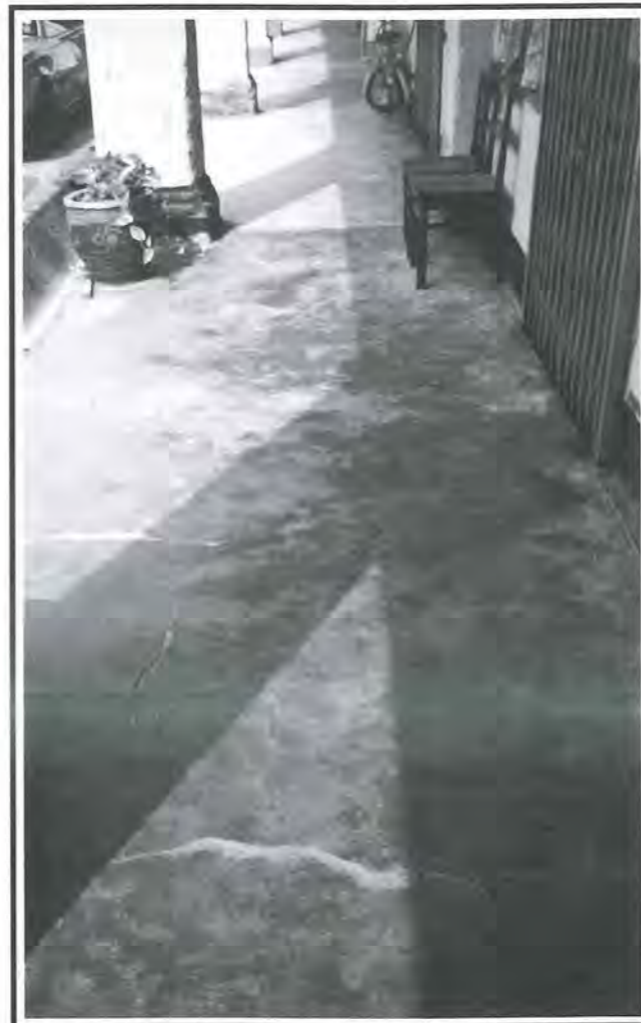
Fig 22: Cracks along the floor indicate settlement of the ground structure and possible damage to the floor slab. In such instances, repair and reconstruction works are usually necessary.
