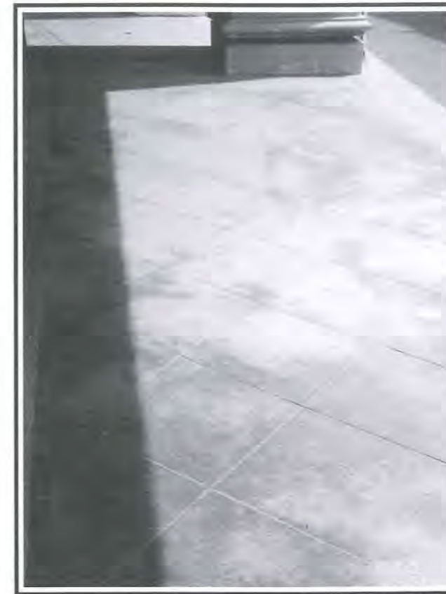
Fig 23: Deteriorated colour cement tiles due to water penetration from the ground.
