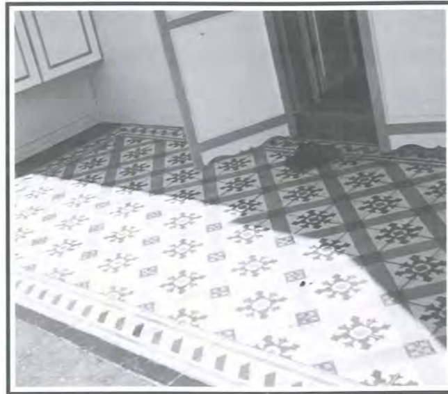
Fig 8: Elaborate use of patterned cement tiles along the five-footway is characteristic of some of the later shophouse styles.
