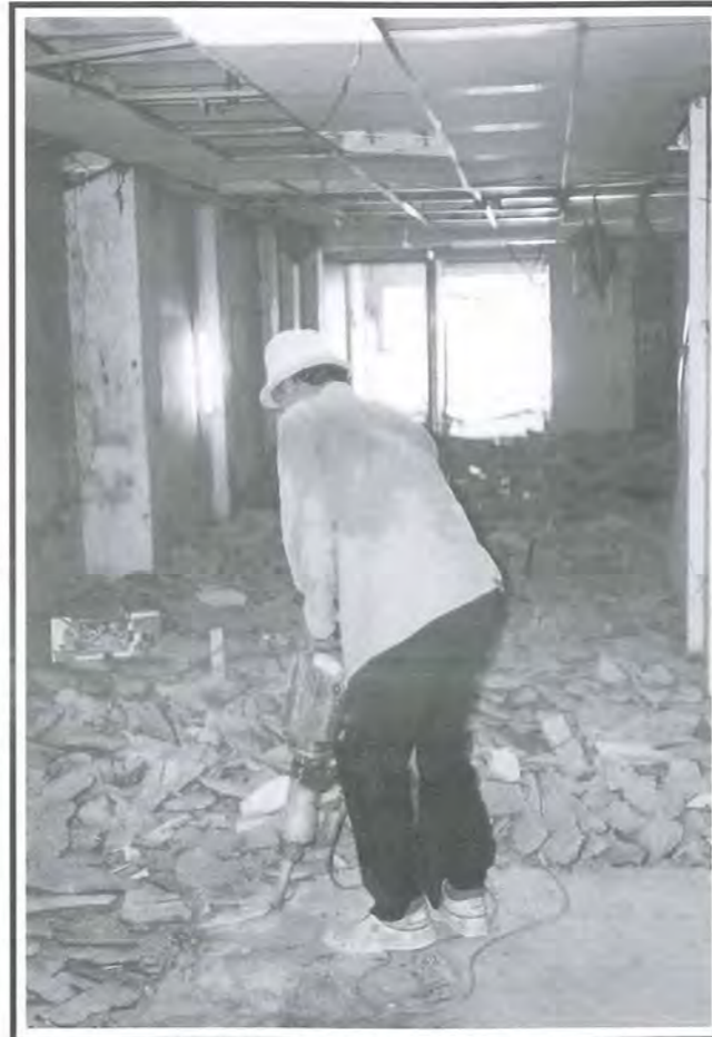
Fig 31: The existing floor slab is demolished in order to facilitate the laying of underground services.
