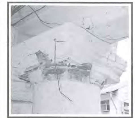
Fig 28: Spalled plaster on the capital of a column.
