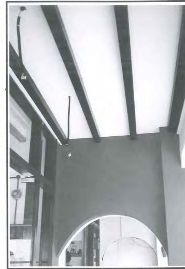
Fig 10: Exposed underside of the upper floor timber joists with the use of plasterboard to conceal the electrical conduits.
