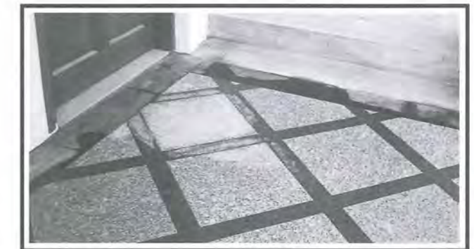
Fig 36: Polished five-footway finishes are potentially hazardous to pedestrians as they are slippery when wet.
