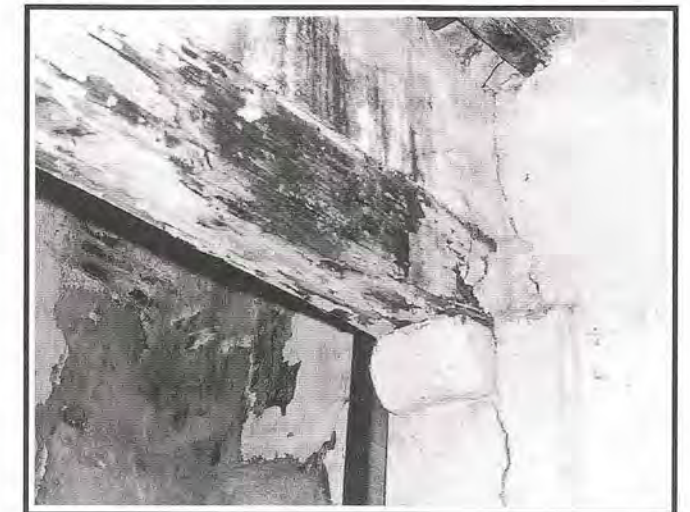
Fig 4: Badly decayed timber door frame.
