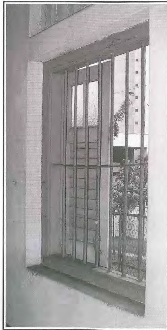
Fig 2: Existing condition of original timber casement window still in relatively good condition.
