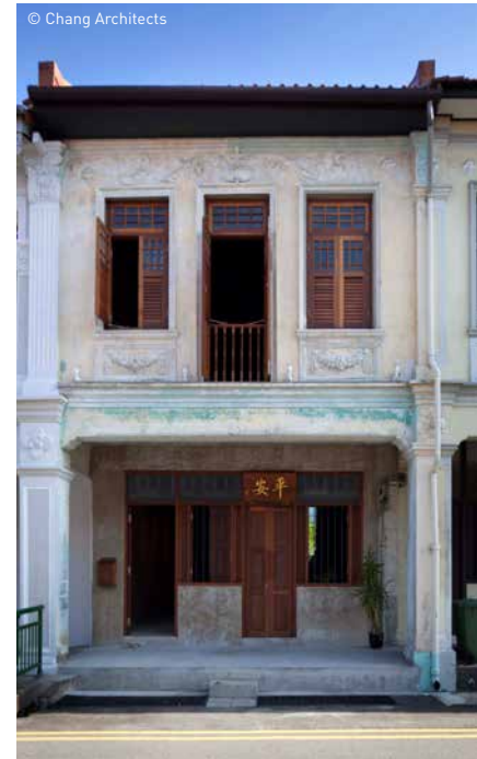
Decorative mouldings on the façade of 125 Joo Chiat Place, formerly the Lucky Book Store
