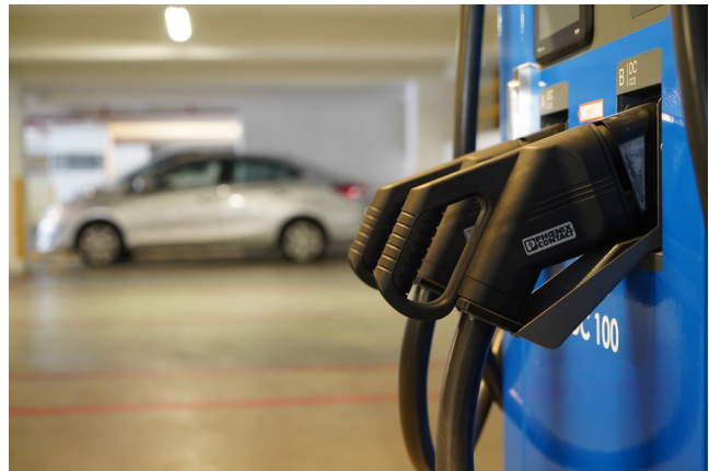
The first EV chargers under the pilot URA-LTA tender were rolled out in public car parks © Ministry of Transport
