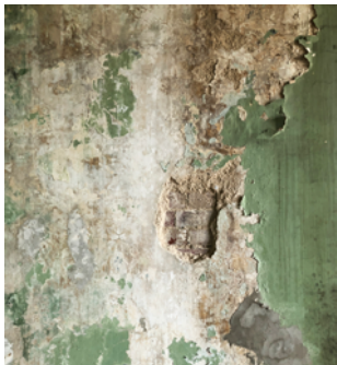
Top: Efflorescence on historic painted mural.
