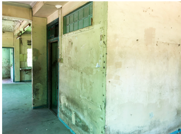
A range of paint degradation observed in this interior space: moisture-related mould growth, blistering, delamination, etc. Buildings left vacant for long periods, or obscured areas (such as behind shelving, above false ceiling), often have aggravated deterioration due to lack of maintenance.
