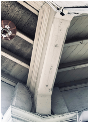
Painted timber ceiling of a shophouse five-foot way – only planks on the left side are mould-infested, indicating a persistent moisture problem.
