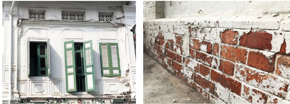
Left: Film-forming paint applied on historic shophouse facade results in extensive delamination, bulging, water retention and plant growth behind the unsightly 'loose skin' of coating. Right: Overpainted historic fairfaced bricks – the unbreathable coating not just obscured the original masonry but also caused its deterioration.
