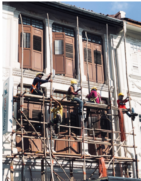
Scaffold being set up for shophouse facade maintenance cleaning, painting and repair works.
