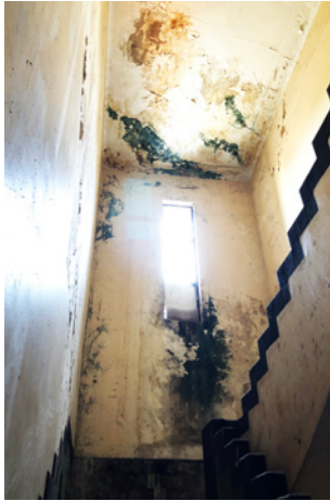
Left unaddressed, rain infiltration through a deteriorated building envelope eventually affects interior finishes and elements – in this case, extensive paint and plaster failure, and mould infestation.
