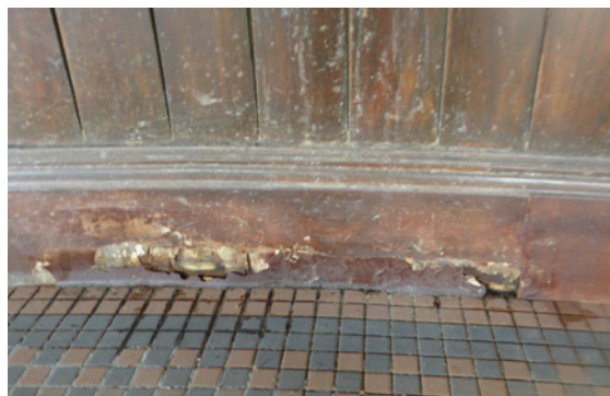
Inadequate and inappropriate maintenance: Wet rot at the timber skirting may have been caused by constant exposure to moisture without sufficient ventilation or time to dry out. It was further painted over, likely to cover the initial stains, leading to trapped moisture and worsening of the untreated rot.
