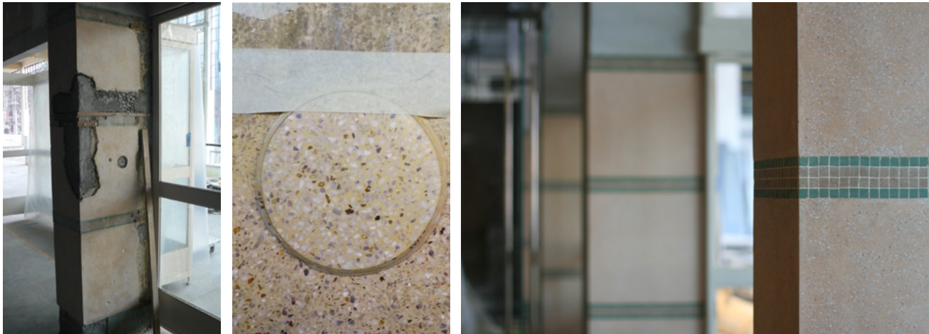
From left: Damaged in situ terrazzo render; one of the patching trials carried out to ensure visual compatibility of patching mix; selected mix is then used for restoring the rest of the terrazzo finished columns.
