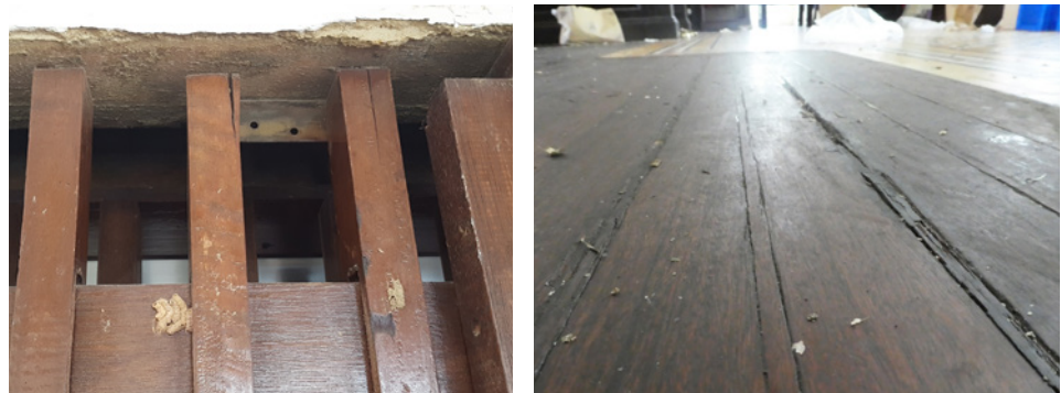
Left: Minor splits at the ends of timber slats and insect infestation. Right: Timber shrinkage due to temperature and moisture fluctuation from air conditioning resulting in gaps between planks.
