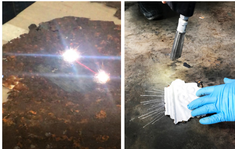
Coating and rust removal using specialist laser (left) and dry ice (right) methods.
