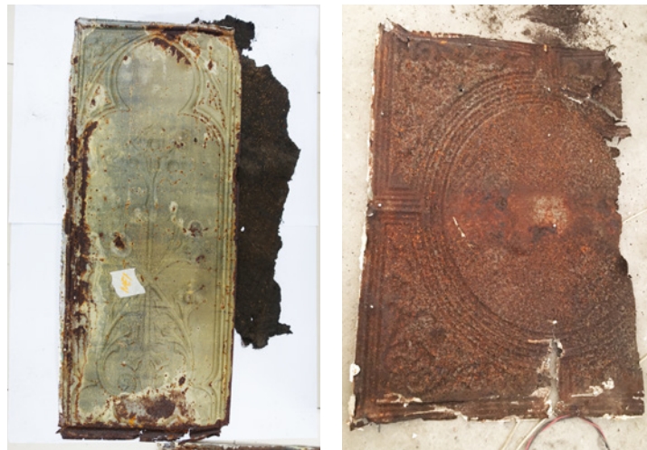
Right: Stamped metal dado panel rusting along the edges. Far right: Panel has completely rusted on the back, which faces the humid, under-ventilated roof space.
