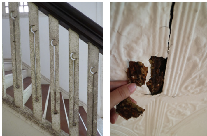
Left: Historic buildings left locked up and unoccupied for long periods become vulnerable to mould infestation in the warm and humid local climate. Right: Severe rusting of ornamented pressed metal ceiling due to moisture from condensation in the roof space arising from the introduction of air conditioning.
