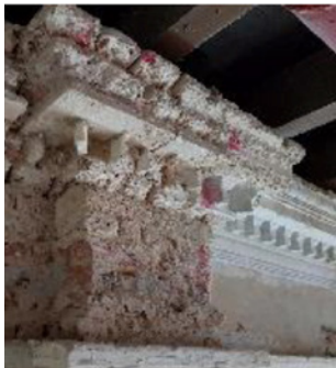
Top: Mock-up for ornamental plaster cornice showing masonry substrate build-up. Above: Exposed brick and terracotta substrate underneath ornamented plasterwork, including the cornice and dentil.
