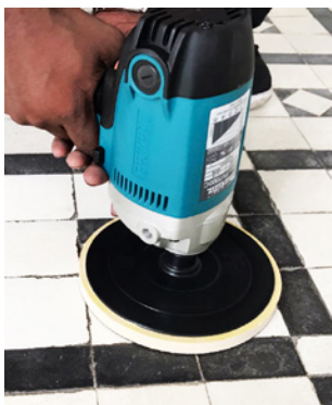
Abrasive cleaning of floor tile using handheld buffing grinder to remove incompatible coating.
