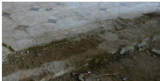
Layers of floor build-up can be clearly seen – finish layer, screed, sand blinding and compacted hardcore.
