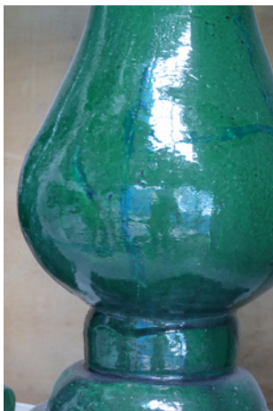
Repair of minor cracks on green glazed bottle balustrade using pigmented epoxy.
