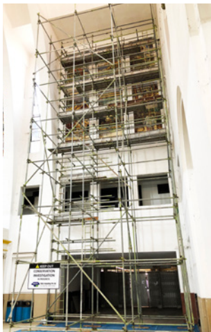
Conservation maintenance inspection using temporary scaffold to access high-level mural wall tiles.
