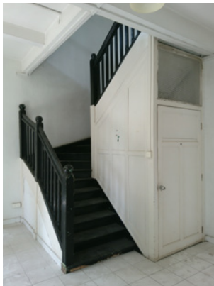
Historic timber staircase with winder steps and storeroom tucked into the undercroft.
