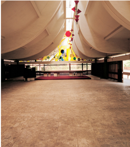
The unusual Cocciame (broken Travertine) floor tiles in the Trinity Theological College chapel (1969), since restored.
