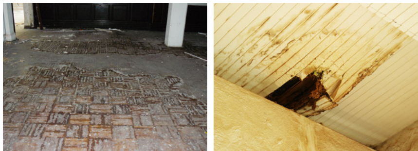
Long-term leakage and ponding on parquet flooring and timber strip ceiling causing extensive damage.
