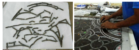
Badly compromised lead comes are dismantled, and localized lead replacement is carried out.
