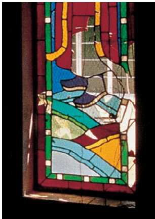
Missing and broken glass pieces on stained glass window.
