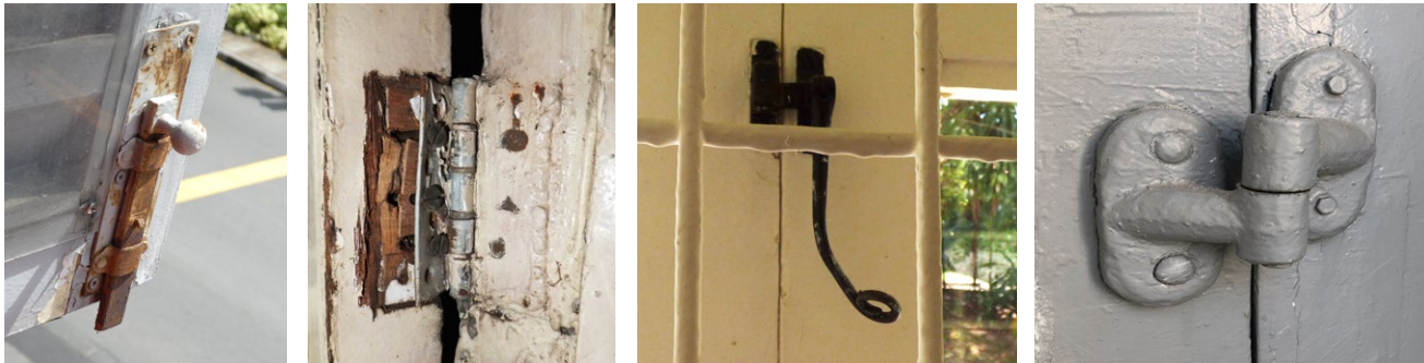
Left to right: Corrosion of window tower bolt; Overpainted, jammed and dislodged butt hinge; Casement fastener with hook handle bent out of shape; Overpainted barrel hinge with mismatched screw fasteners probably from past inappropriate replacement.
