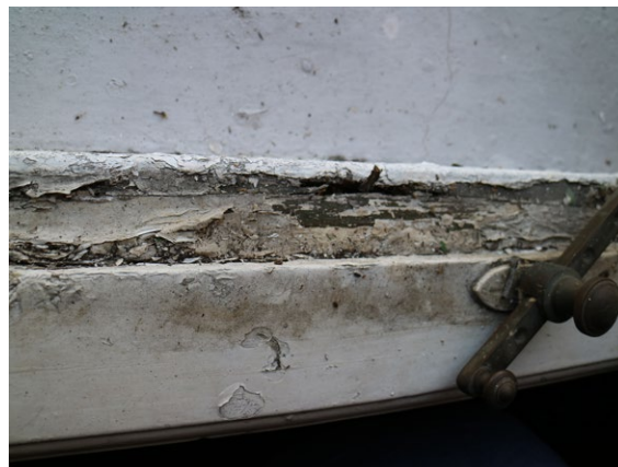
Far left: Dislodged louvres, wet rot and rusted ironmongery.
