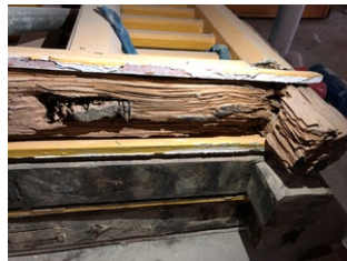
Termite attack in timber components leaving extensive trails.
