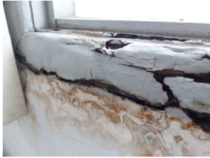
Advanced wet rot and termite infestation observed in timber window sill as a result of deteriorated weather seal and poor maintenance.
