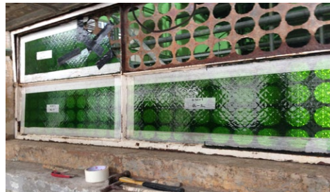
Taping the edges of glazing panels for protection prior to taking down the windows for dismantling the glass.
