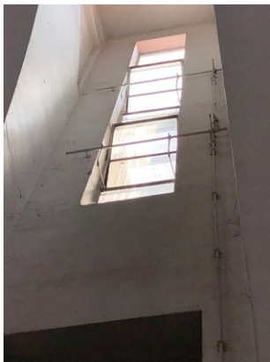
Fenestrations located at heights beyond the reach of ladders pose maintenance challenges, such as these mild steel operable clerestories.
