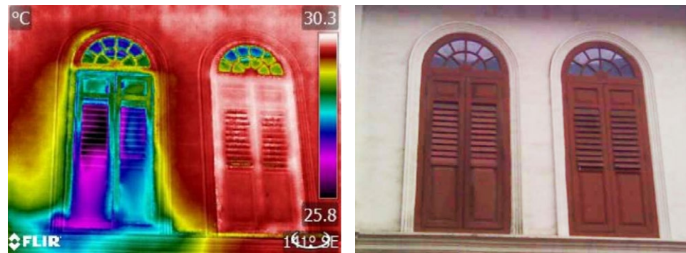
The thermogram shows cold air leaking from the left window, likely due to sealant failure of the interior secondary window glazed panel.
