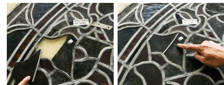
A crack through a major painted glass piece is repaired using string lead, rather than replaced.
