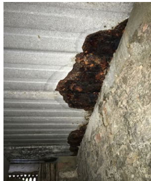
Corrugated steel form and concrete composite slab with water seepage, paint failure, and steel corrosion occurring at the slab-to-wall junction.
