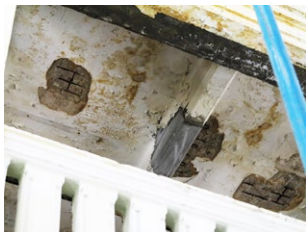
Patch repair to RC beam spalling at midsection, prior to plaster and paint finishing.
