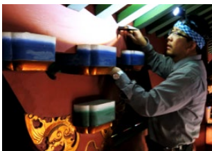
Master carpenter conducting visual and tactile survey on the traditional timber structures at Shuang Lin Monastery.
