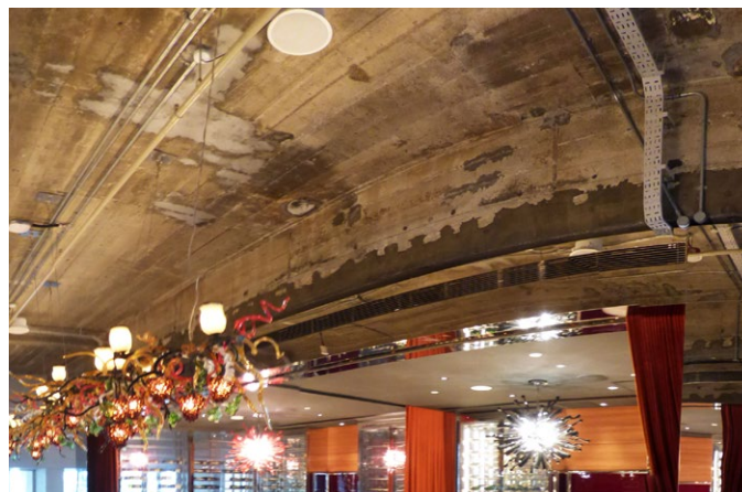
Existing RC beam strengthened through increase in sectional depth by casting of new high-strength concrete beam below (note darker material along the bottom of the beam).
