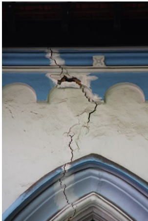
Visible sign of structural defect – crack through arch structure.
