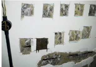
From top: Surface hardness test on concrete using rebound hammer; measurement of half-cell potential to gauge degree of concrete deterioration.
