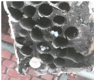
From top: Dilapidation – displaced timber truss joint; termite trails along timber beam and wall around beam end; after damaged by carpenter bee infestation.
