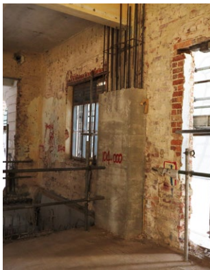
Addition of RC column to support existing beam and stiffen the masonry wall.
