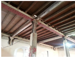
Breakout of a latter-day concrete encasement to reveal the historic steel structure originally designed to be exposed.
