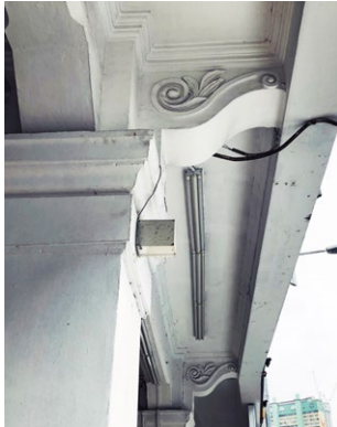
Ornamental facade RC feature corbels that may be adversely affected if strengthening is applied.
