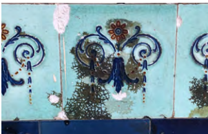
Top: Historic mosaic tiles uncovered after removal of insensitive latter-day cladding works. Above: Cracking in the surface glaze resulting in moisture ingress through the glaze. Over time, mould growth has occurred within the cracks.
