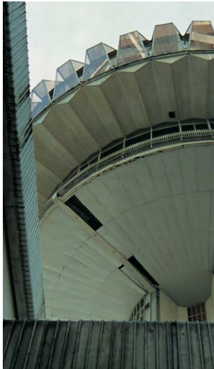
Multiple signs of damage in the metal cladding, including missing units, warpage, dislocation, staining and corrosion.
