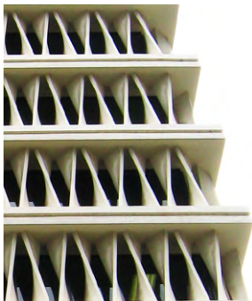
Top: Breathable facade screen wall at SGH Housemen's Quarters (1950s). Above: Wing On Life Building (1975) - precast 'twisted' RC panels doubling as screen wall and structure.
