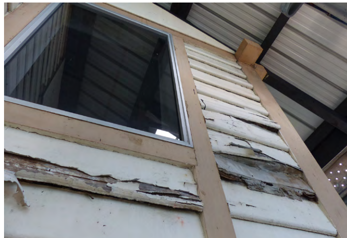
Deteriorated timber siding and poorly executed ad hoc repair using incompatible material.
