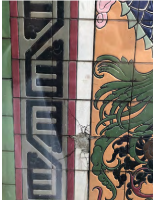
The first stage of diagnosis involves a visual survey and mapping of observable defects such as cracking.
