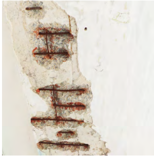
Exposed reinforcement of spalled concrete is cleaned and treated with anti-corrosion coatings, before replacement grout is applied.
