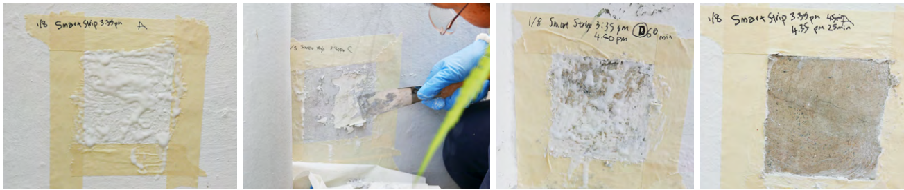
The images above show the sequence of application of ecofriendly paint stripper, combined with manual scraping, for removal of paint over plastered finishes.
