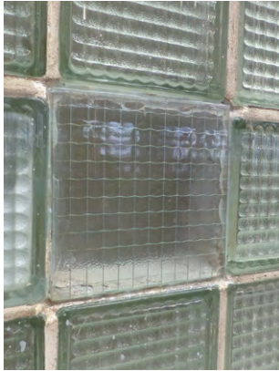
Latter-day ad hoc 'replacement' using a piece of wired glass. Missing blocks should instead be inserted with a matching replacement unit to restore not just the appearance but also structural integrity of the glass block wall.
