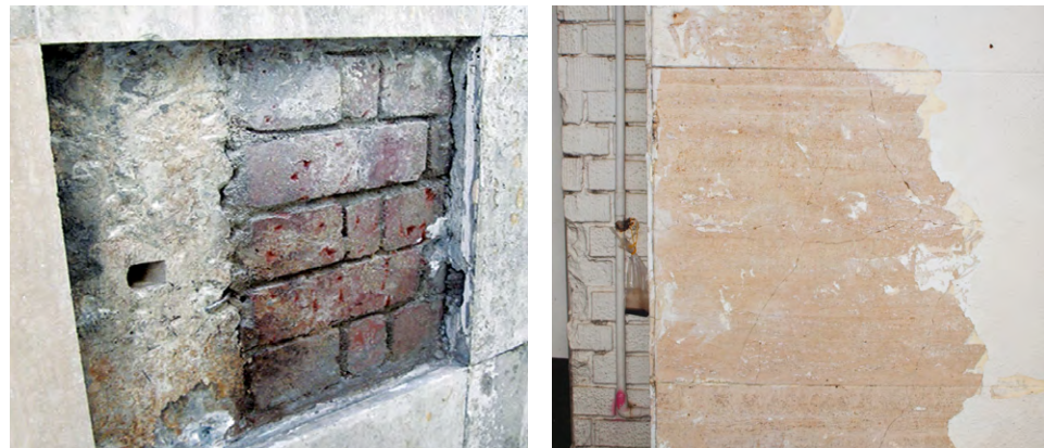
Left: Water ingress through mortar joints can affect the adhesion of the panel to the substrate, resulting in debonding. Right: Cracks on the panel near the frame, possibly arising from movement of the building.
