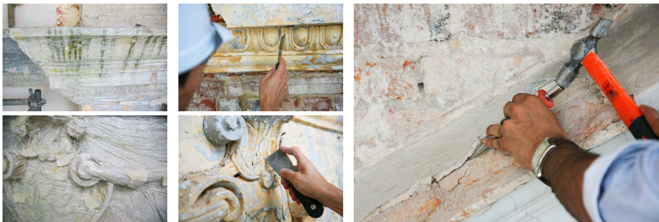
Left: Removal of paints by application of chemicals on the surface. The surface is wrapped in plastic to improve the chemical softening of paints. Middle: Manual paint removal for delicate relief details. Right: Removal of incompatible cementitious layers by chiselling.
