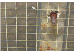
Some defects can be manmade, such as insensitive renovation works to install services.
