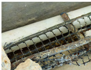
Plaster rendered on metal mesh substrate ( above ) for lightweight parapet wall ( top ) at the former Traffic Police Headquarters.
