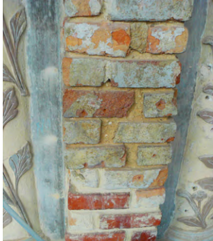
Brick substrate exposed after removal of incompatible plaster render at Stamford House.
