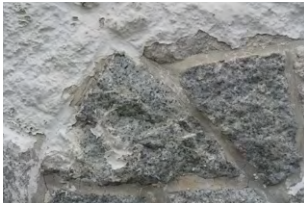
Paint coatings obscure the stone surface and other conditions.
