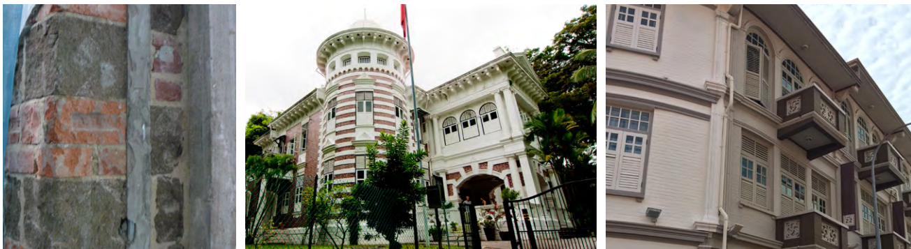
Left: Hybrid masonry walls constructed from brick and concrete blocks. Middle: Golden Bell Mansion at Mount Faber, constructed in an alternating combination of fairfaced and plastered brick popularly known as the "blood-and-bandage" style. Right: Shophouse with fairfaced brick facade painted over. The original texture, colour, and character of the building has become obscured and homogenized.
