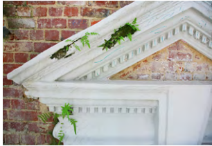
Plant growth on facade ornamental plaster mouldings.
