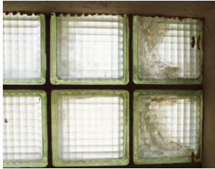
Stains on the internal surface of the glass blocks, possibly due to infiltration of moisture through cracked or broken mortar joints.
