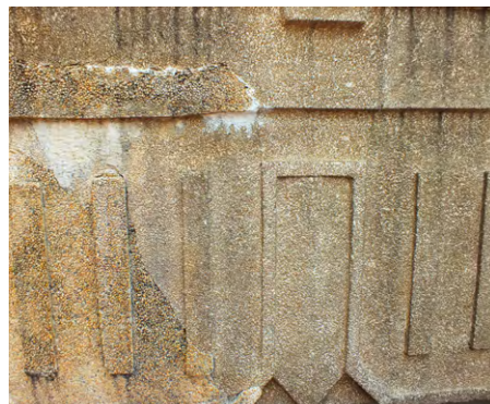
Incompatible patching using modern-day pebblewash, which appears incongruous against the historic Shanghai plaster. The white 'stains' along the patch lines are salts efflorescence arising from water ingress through the seams.
