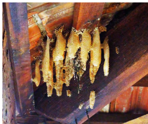
Wasp nest under roof eave.
