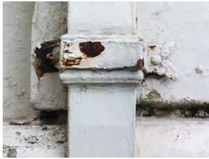
Top: Gutter choked by dead leaves despite having been installed with a wire mesh cover, leading to plant growth. Above: Paint peeling and badly corroded bracket securing downpipe to wall.
