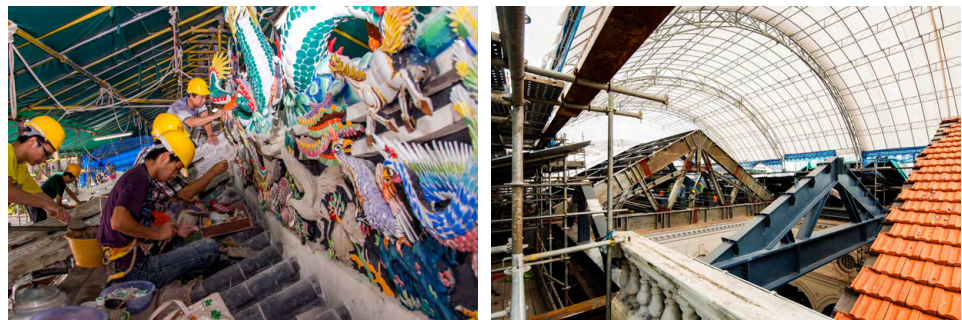
Left: A simple pole-and-canvas temporary roof for restoration of delicate temple ceramic shardwork at Wak Hai Cheng Bio. Right: Mobile temporary roof mounted on tracks that can be moved according to the roof section undergoing works, at the Victoria Concert Hall.
