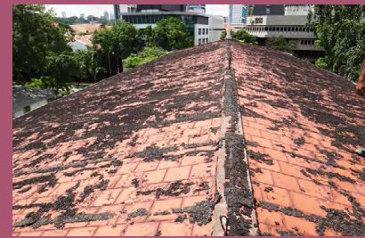
The topmost bituminous waterproofing membrane of the RC roof slab has badly deteriorated, revealing the underlying terracotta tile layer.
