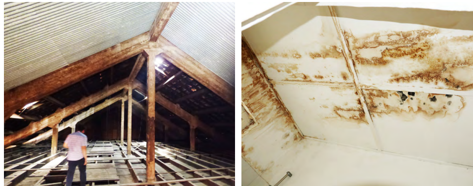
Left: Inspection of roof space between ceiling and roof covering. Right: Water ingress through defective roof causing ceiling stains and deterioration.
