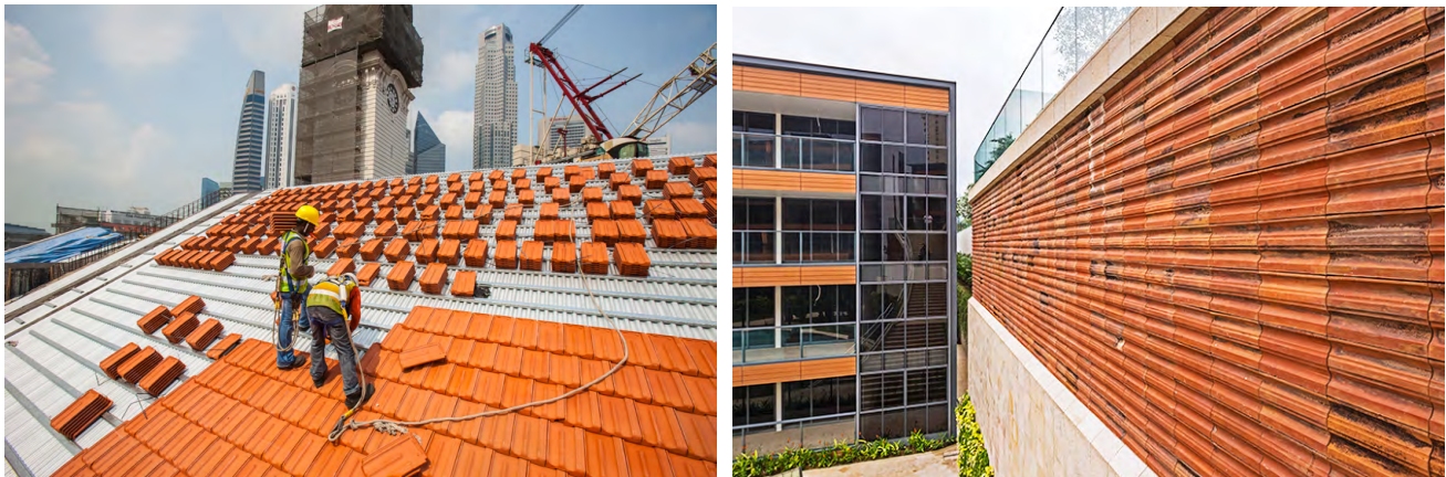
Left: Corrugated metal deck as secondary roof receiving galvanised steel battens and Marseille tile finish, at the Victoria Concert Hall. Right: Salvaged historic Marseille roof tiles upcycled as landscape feature wall in the adaptive reuse development Sophia Hills.
