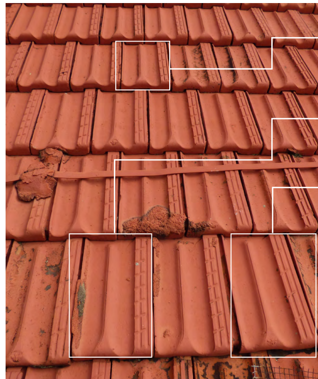
Three different brands of Marseille found on the same roof plane, identified by the different imprinted brand logos.
