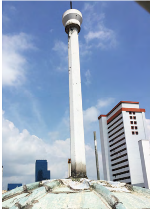
Corrosion, paint peeling and staining observed around the anchor point and joints of a metal flag post mounted atop a copper dome roof.
