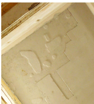
Concrete rehabilitation by integration repair—white patches of fiber-reinforced mortar applied on badly spalled RC roof slab to return strength and integrity to the concrete cover.
