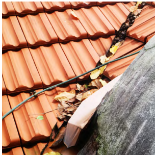
Leaf litter choking up roof valley gutter – unreachable areas such as this may only be detected with elevated access or via a drone recording.
