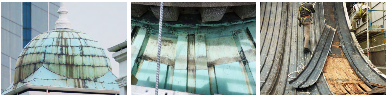
Left: Iron rust run-off on copper roof. Middle: Inconsistent erosion of patina layer and stain accumulation due to different exposure, run-off of water and effect of pollution. Right: Termite attack in the timber backing below the galvanised steel roof sheets and insulation felt/fabric.
