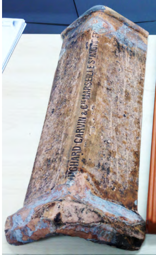
Weathered ridge tile showing surface erosion, chipping, cracks and flaking.
