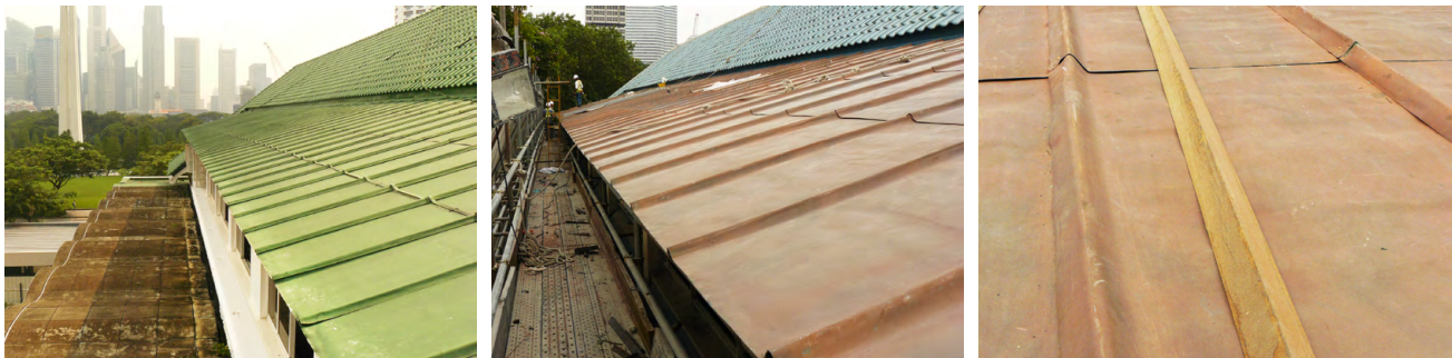
Left & middle: Inappropriately painted copper pitch roof – before and after paint removal. Right: Deteriorated roof sheets were selectively replaced – photo shows timber strip used for manually forming the triangular profile standing seams.
