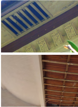
Top: Timber board eave soffit with a ventilation panel. Above: Exposed timber ceiling joists on which the timber strip ceiling (as seen on the left) was secured.
