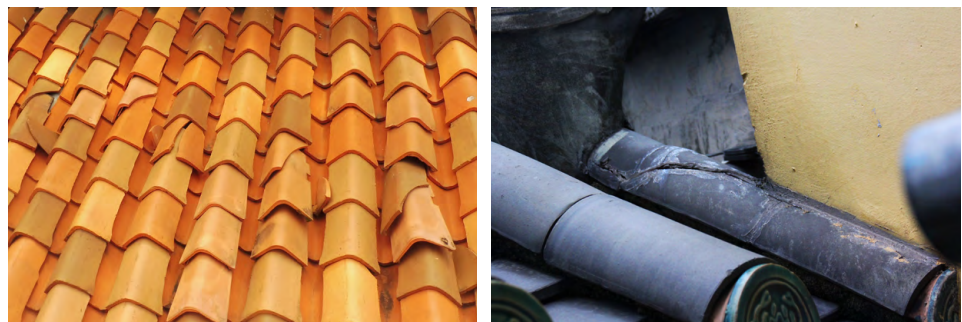
Roof tile breakage
