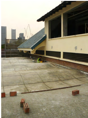
Applying finishing screed to restored thin shell RC vaulted canopy. The original roofing did not have a waterproofing layer, and adding one would have changed the thin-shell roof aesthetics – instead a waterproofing additive was added to the finishing screed.
