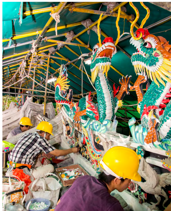
A temporary roof is erected while skilled artisans are flown-in to undertake the delicate and painstaking work of restoring rooftop qianci at Wak Hai Cheng Bio.
