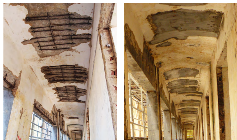
Repair of RC roof concrete spalling – removal of deteriorated concrete and rust, replacement of rebar if necessary, treat with anti-rust coating, and patching with compatible mortar.
