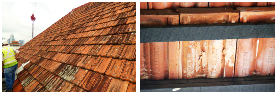
Left: Eroded tile surface and biological growth. Right: Efflorescence, or salt crystallization on roof tile – due to the clay tile body containing high salt content.
