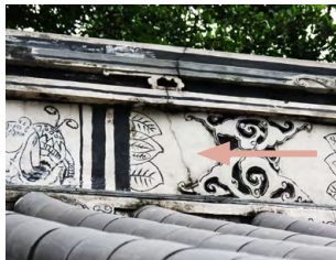
Crack line across ridge beam of a traditional Chinese roof indicating structural distress.
