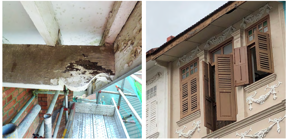
Left: Paint peeling and wet rot of fascia board and supporting rafter end. Right: Deteriorated shophouse fascia and soffit.
