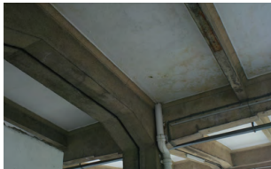
Water seepage stains and efflorescence at the undercroft of RC roof slab.
