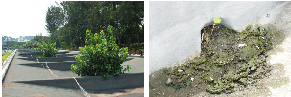
Left: Plant growth on RC roof canopy where the drainage holes are located suggests that there is chokage – any debris should be cleaned, and vegetation growth carefully removed and treated with herbicide. Right: Accumulation of dirt, debris and plant growth at the drainage holes of an under-maintained flat roof.
