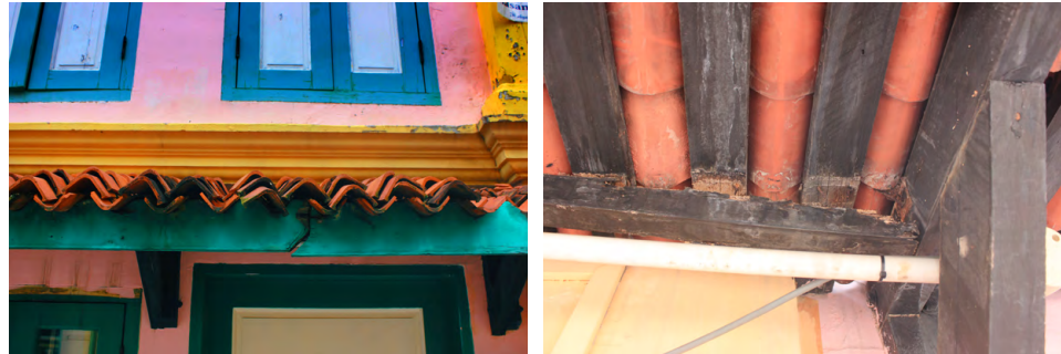
Deterioration and dislocation of v-profile tiles, disjointed roof timber members suffering from wet rot and structural risk – defects that should have been detected and addressed in their early stages by regular maintenance were instead left to worsen.
