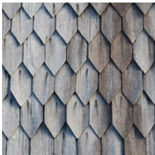
Streaking and discolouration resulting from exposure to rain and pollution.
