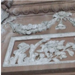
Radiation and exposure to rain results in fading of painted surfaces.
