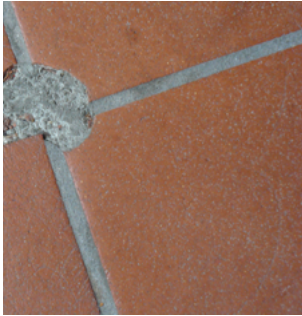
Tiles with minor chipped edges can be left in place, since it will be costly to repair the tile, with very minimal visual benefit.
