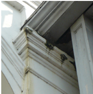
Moisture-induced damage often occurs at joints and cracks on external wall finishes, bridging at insulated walls, open joints, penetrations through walls, roof and basement, rainwater collection points, and windows.
