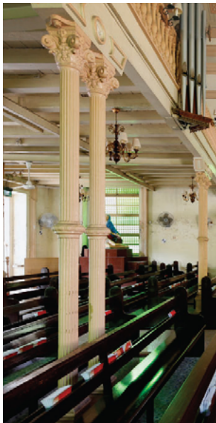
Cast iron columns supporting the choir loft at the Cathedral of Good Shepherd
