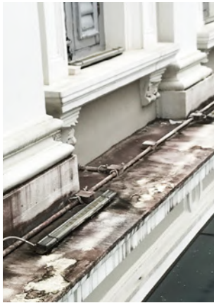
Eroded projecting ledge resulting in water ponding and staining of the facade. If left untreated, there will be increased risk of rainwater seepage into the interior.
