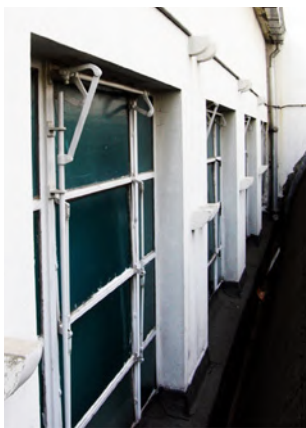
Exterior view of mild steel windows at the courtroom mezzanine, prior to restoration.
