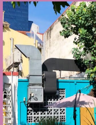
Uncoordinated kitchen exhaust flues penetrating rear facade elements and causing visual clutter.
