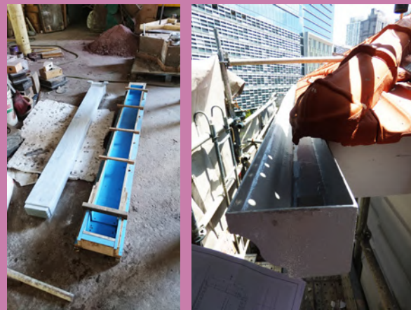
Left: A newly cast segment of rainwater downpipe. Right: Newly installed gutter. The repaired and replaced cast iron goods are treated with anti-rust coating and paint to protect them from deterioration.
