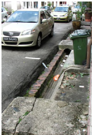
Prior condition of street interface with uncovered drain and uneven pavement levels.
