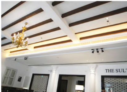
Main lobby with exposed timber ceiling joists. Drop ceiling is kept to one end, with false ceiling selectively installed between joists where needed to accommodate services and lighting.
