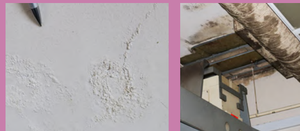
Moisture presence resulting in salt attack (left), mould growth (right) and poor indoor air quality.
