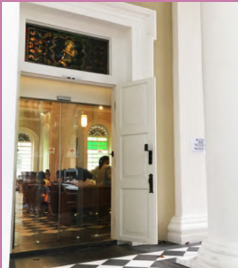
Secondary frameless glass automated sliding doors are added behind the restored historic doors, which are held open during operating hours.
