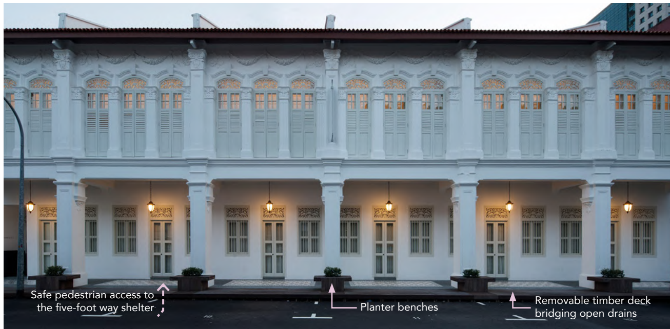
Timber deck and planters were introduced along the front of the Aliwal Street wing.
