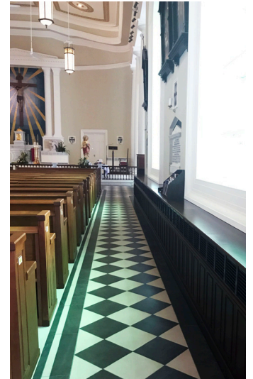
Air-conditioning units sensitively hidden behind cabinets
