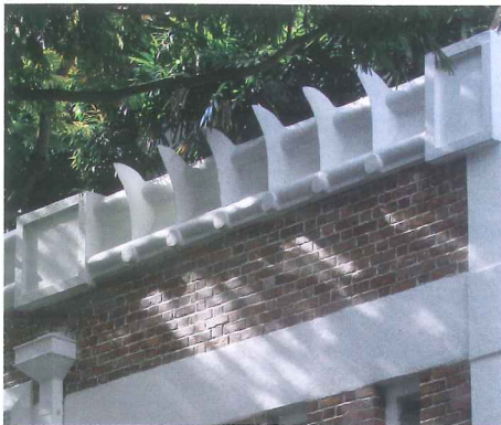
Claw-like protrusions repaired
