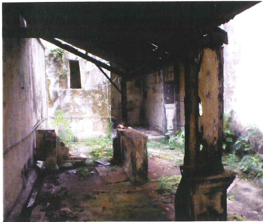
Courtyard before restoration showing years of neglect and dilapidation
