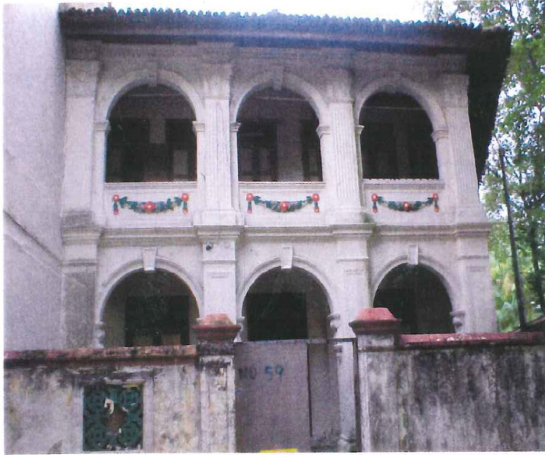
Façade of 59 Blair Road before restoration. The boundary wall on the left was so structurally unsound, it fell soon after this picture was taken. See picture at right
