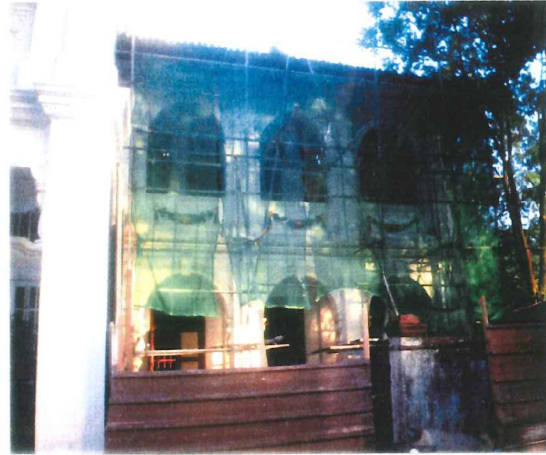
Façade showing collapsed left boundary wall
