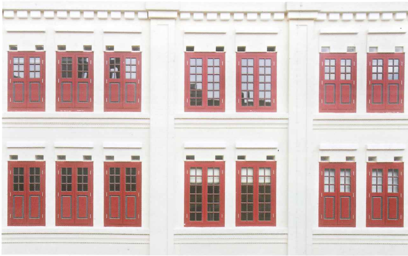
Character of external facade with original vents and windows retained and restored
