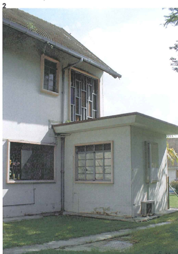
Exterior View of the staircase wing connecting the first storey with the second storey
