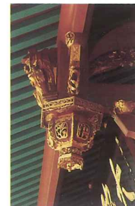
Timber hanging post
