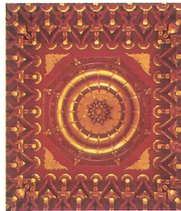
Restored ceiling at Da Xiong Bao Dian
