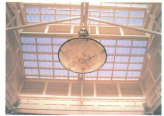
New light fitting under skylight over triple-volume atrium
