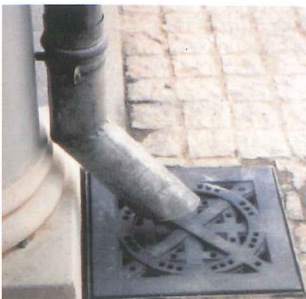
Grating over drain
