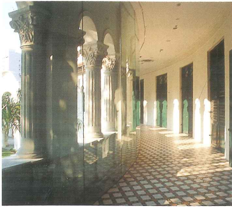
Restored Corinthian columns and their plaster works kept intact by using detached sheet glass, thereby retaining the spatial quality and character of the colonnaded passageway
