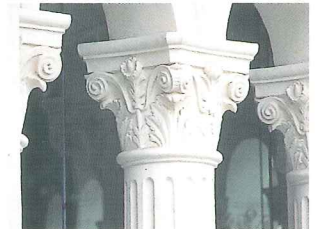
Fine cementitious grout injected to re-bond delaminated plaster on Corinthian columns to preserve the craftsmanship of 1903
