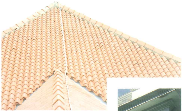
Natural colour unglazed V-profile clay tiles restored to original height, profile and pitch
